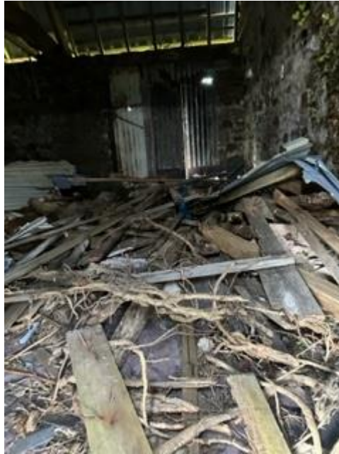
Figure 25 Debris to right hand room.
