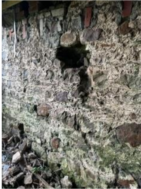
Figure 17 Internal deterioration to internal wall
