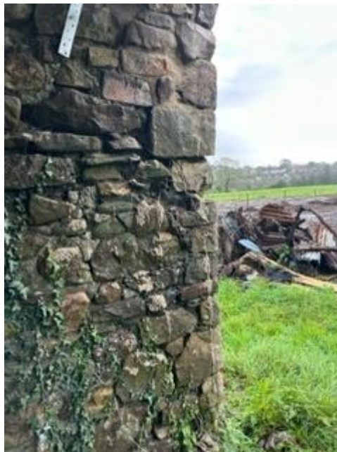
Figure 12 Deterioration to gable end - internally
