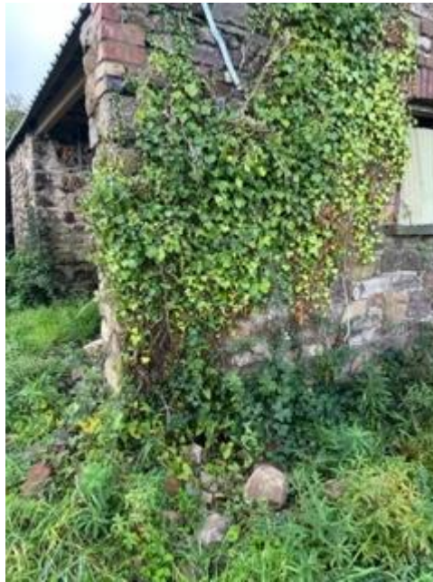
Figure 9 Close up of low-level masonry deterioration
