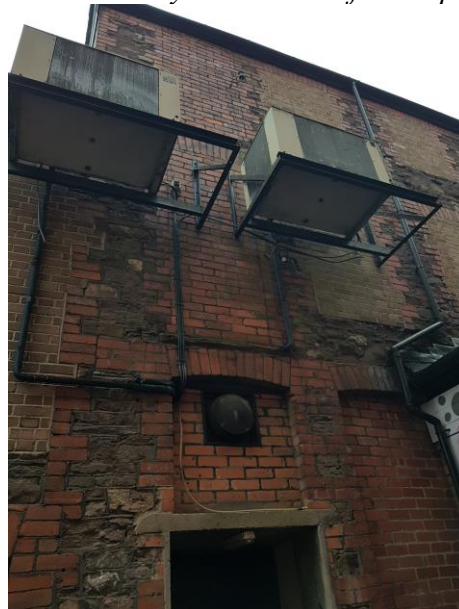
Plate 6 – McCarthy's Court – existing flues and air con units
