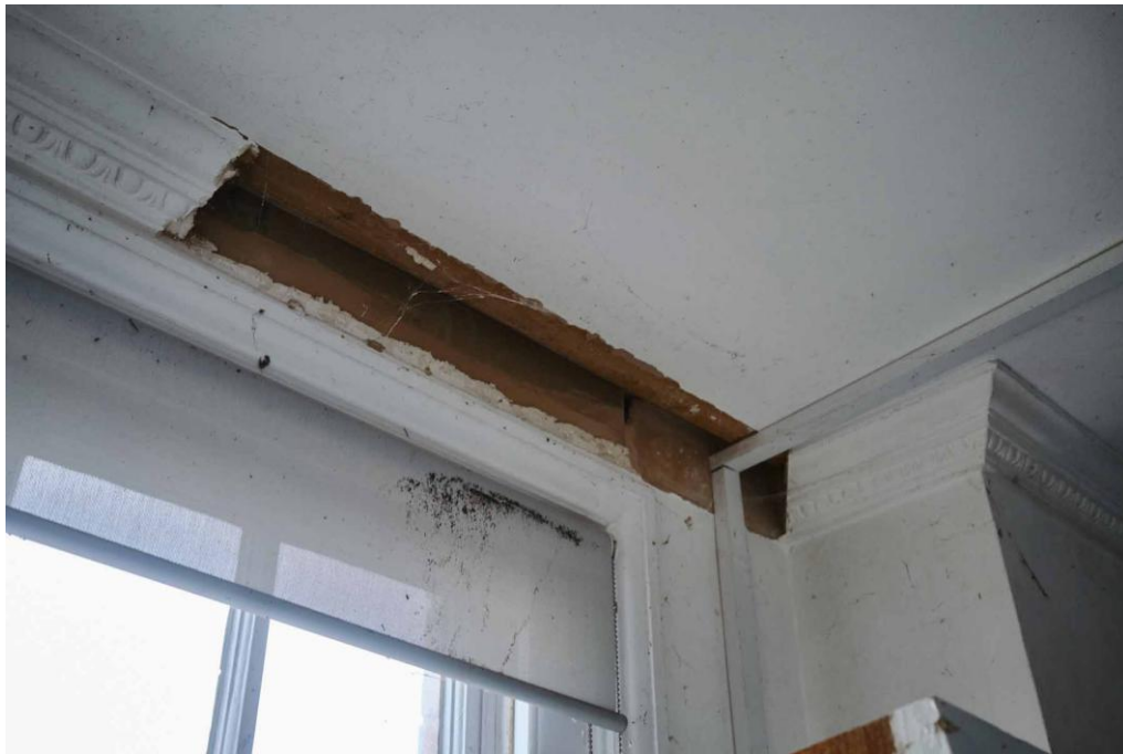
Figure 15. Example of damaged egg-and-dart cornice.
