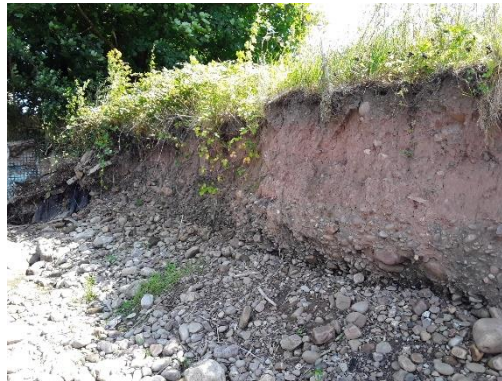
Figure A.35: Example of eroded bank at unprotected downstream area of Reach 4.
