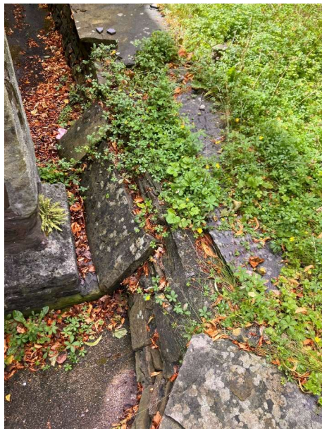
Condition of ledgers at NW corner of North Aisle.
