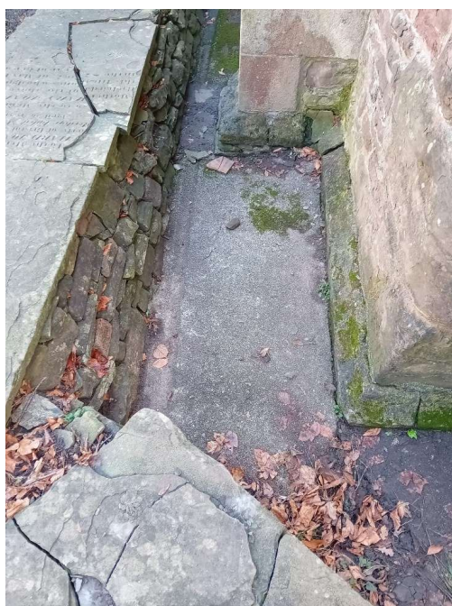
Example of broken ledgers at edge of drainage channel and condition of retaining wall beneath.
