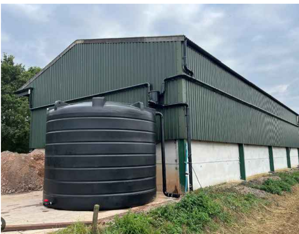
Rain Water harvesting tank with filter.
