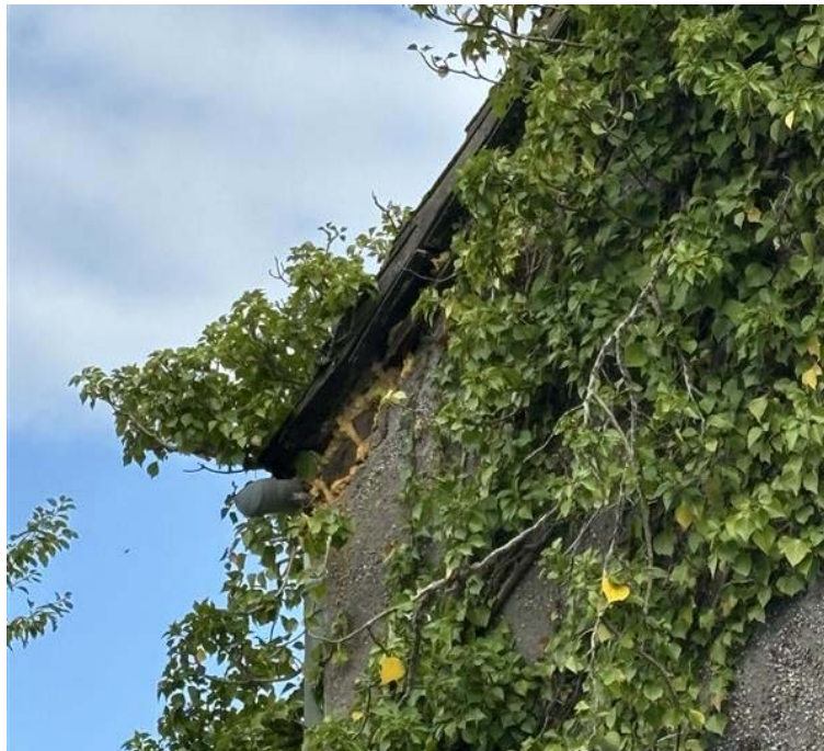
Plate 3 Infilled crack in wall, surrounded by dense ivy cover
