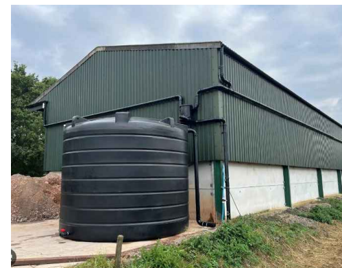
Rain Water harvesting tank with filter.
