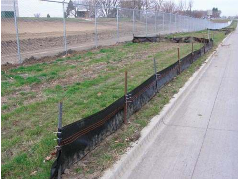
J-hooks create ponding area for sedimentation.
