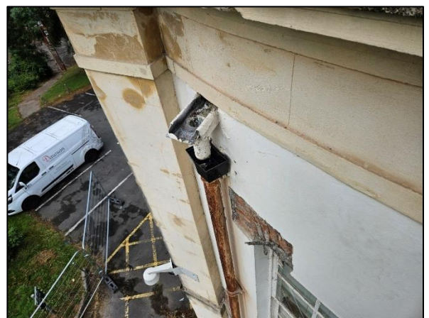
Figure 4-12 - Gutters and Downpipes Corroded
