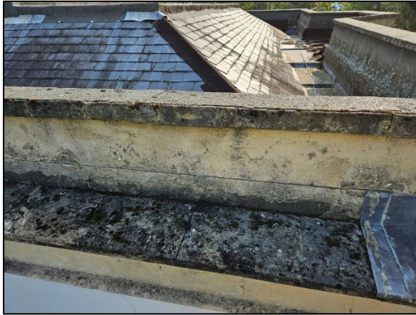
Figure 4-7 - Lead Lining Missing
