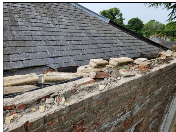
Figure 4-4 - Dislodged Coping Stones
