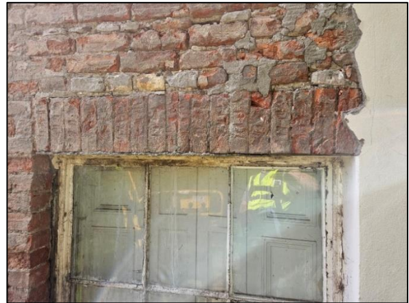
Figure 4-2 – Corrosion on Steel Lintel
