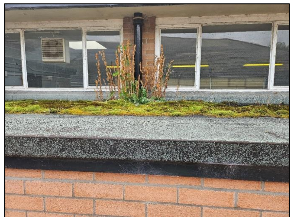
Figure 4-16 - Growth and Ponding on Flat Roof
