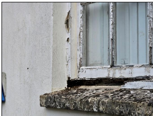
Figure 4-9 - Bees Nest Entrance in Rotten Window Frame
