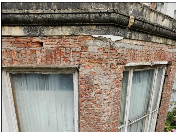
Figure 4-3 - No Arched Brick Soldier or Lintel
