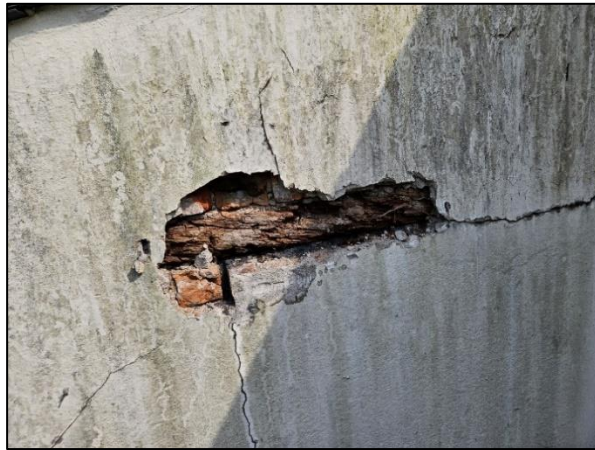
Figure 4-13 - Rotten Timber in Wall
