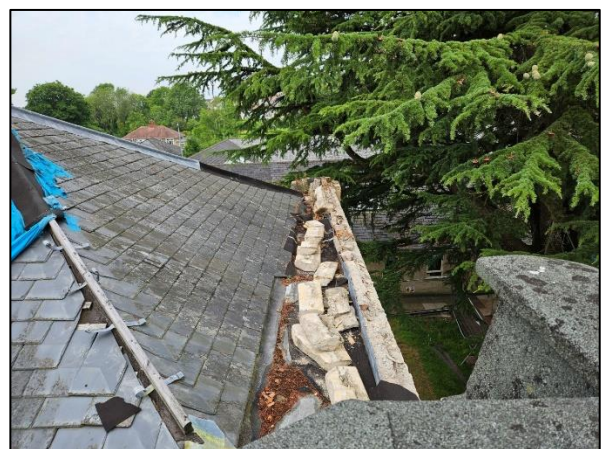
Figure 4-10 - Coping Stones in Poor Condition
