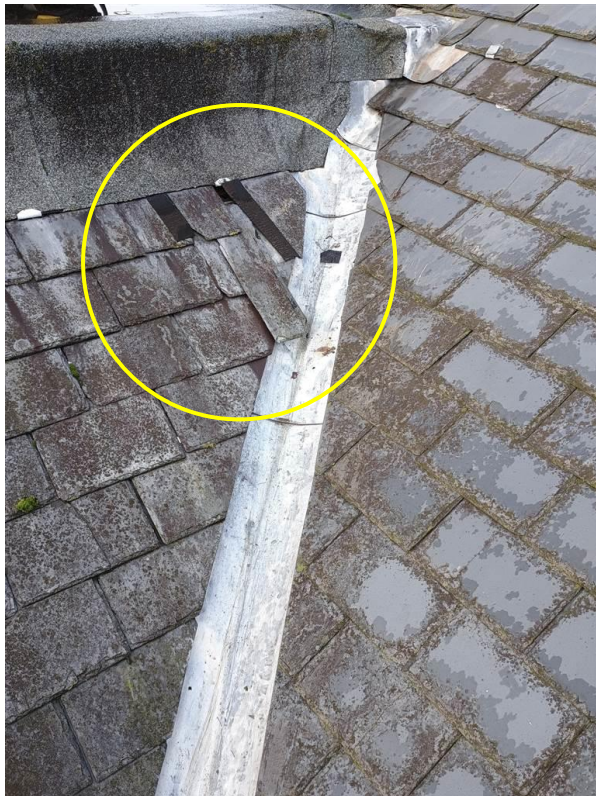
Left: typical view of slipped slates
