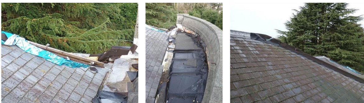
Left: Typical views of stolen lead and temporary repairs, which are now failing
