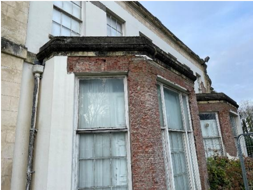
The existing brickwork is inadequate and should be repaired/repointed.
