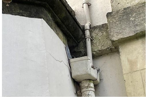
The existing rainwater goods are in poor condition and should be replaced during the refurbishment.
