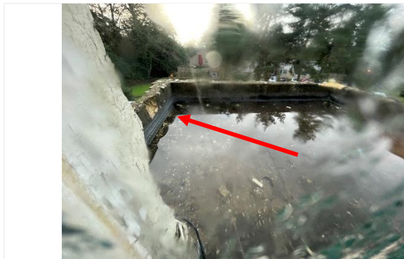
The existing parapet wall is significantly damaged. This should be encapsulated by the new waterproofing.
