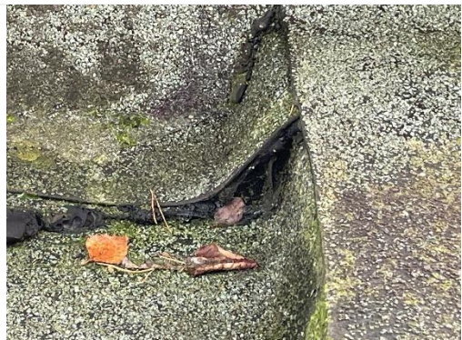
Certain sections of the detailing have started to debond. If not addressed, they will inevitably lead to water ingress.
