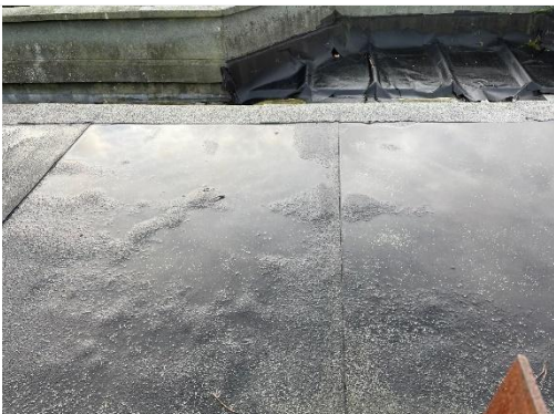
Blistering is visible throughout the roof, indicating raised areas where adhesion between layers has been lost due to trapped air and/or moisture. These pockets expand as the temperature increases. Before refurbishment, all blisters will need to be cut out.
