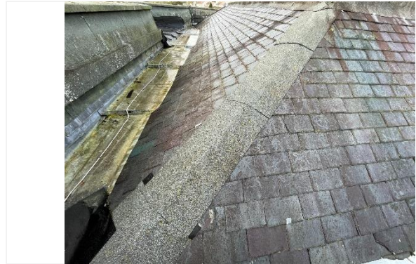
Damaged sections of the pitched roof area are to be included within the scope of works. Lead or appropriate replacement tiles is to be used.
