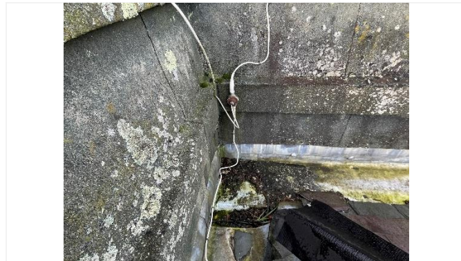
Redundant cables should be permanently removed from the roof area.
