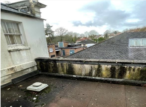
Overview of Roof B - The current system has reached the end of its serviceable life. The redundant mushroom vent should be removed from the roof prior to the commencement of works.
