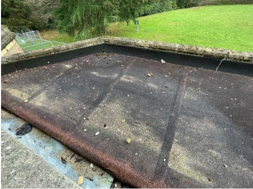
Overview of the existing roof area. The current system has reached the end of its serviceable life.
