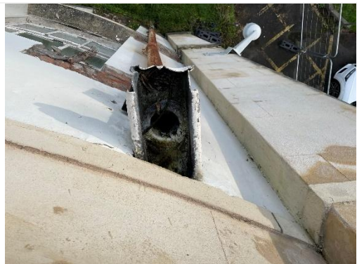
The existing rainwater goods are in poor condition and should be renewed during the refurbishment.
