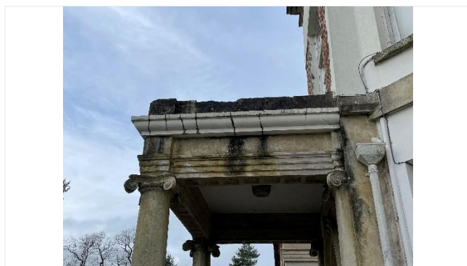
The external gutters are in poor condition and should be removed and replaced during the refurbishment works.
