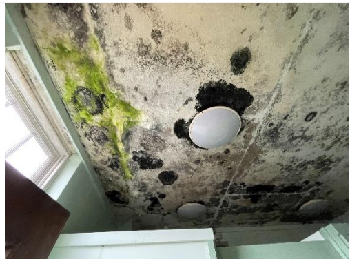
Further evidence of water ingress.
