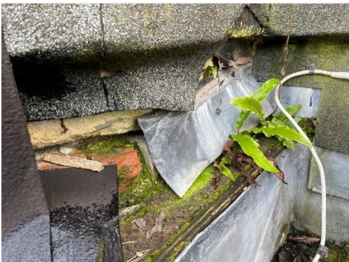
The existing detailing is poor.
