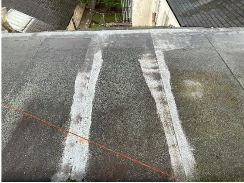
Liquid repairs are evident across the roof area, these should only be considered as short-term solution.
