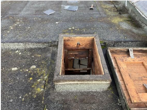
The access hatch will need to be re-detailed and cover reinstated, as part of the scope of works.
