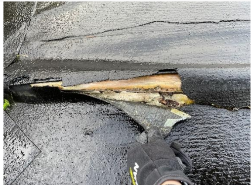
Large scale temporary repairs were installed, but these have now started to fail re-exposing the issue.
