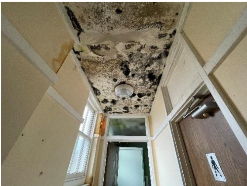
Significant water ingress has caused mould to occur. This indicates that water is penetrating the current waterproofing.
