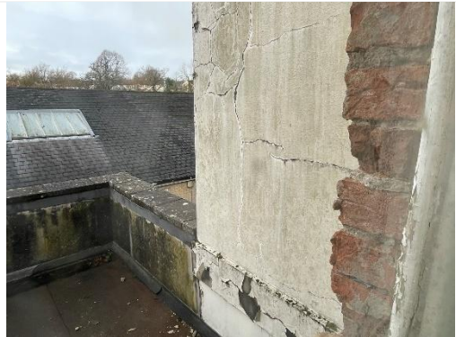
The damaged render is likely contributing to water ingress and should be replaced as part of the re-roofing works to ensure a watertight and durable finish.
