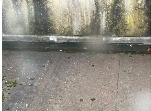
The internal gutter is holding a significant amount of ponding water. Regular maintenance should be implemented to prevent any future blockages.
