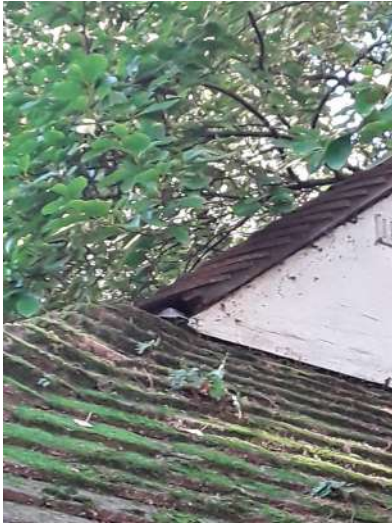
Photograph 19: lifted roof tiles and within brickwork of Building S2.
