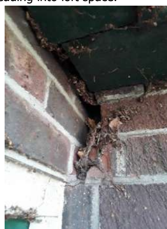
Photograph 18: Birds nest and crack within brickwork of Building S2.
