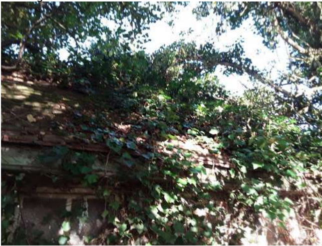
Photograph 21: Ivy covering building S2's roof
