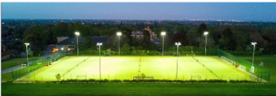
Figure 7 - LED Floodlighting System
