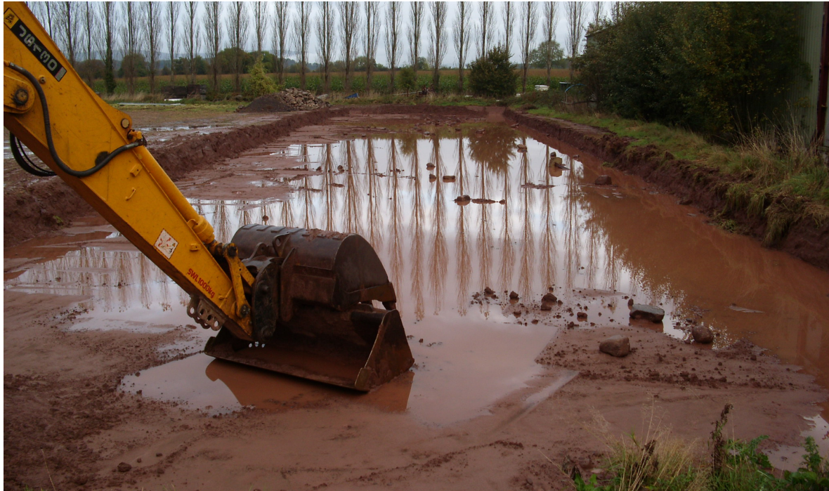
Photo showing the current amount of topsoil imported to our site from this location.
