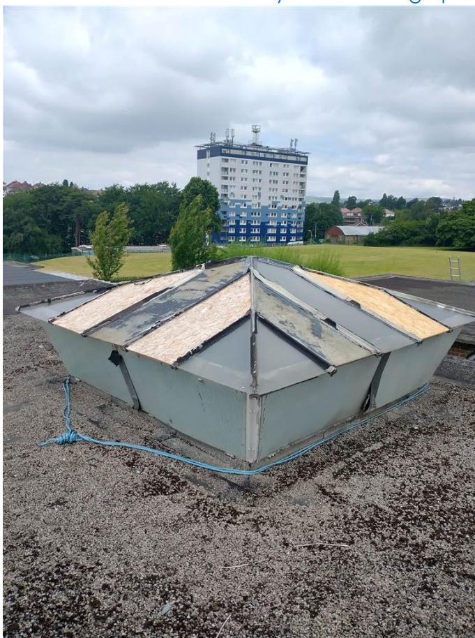
Left: Typical image of the lantern's poor condition (2024)
