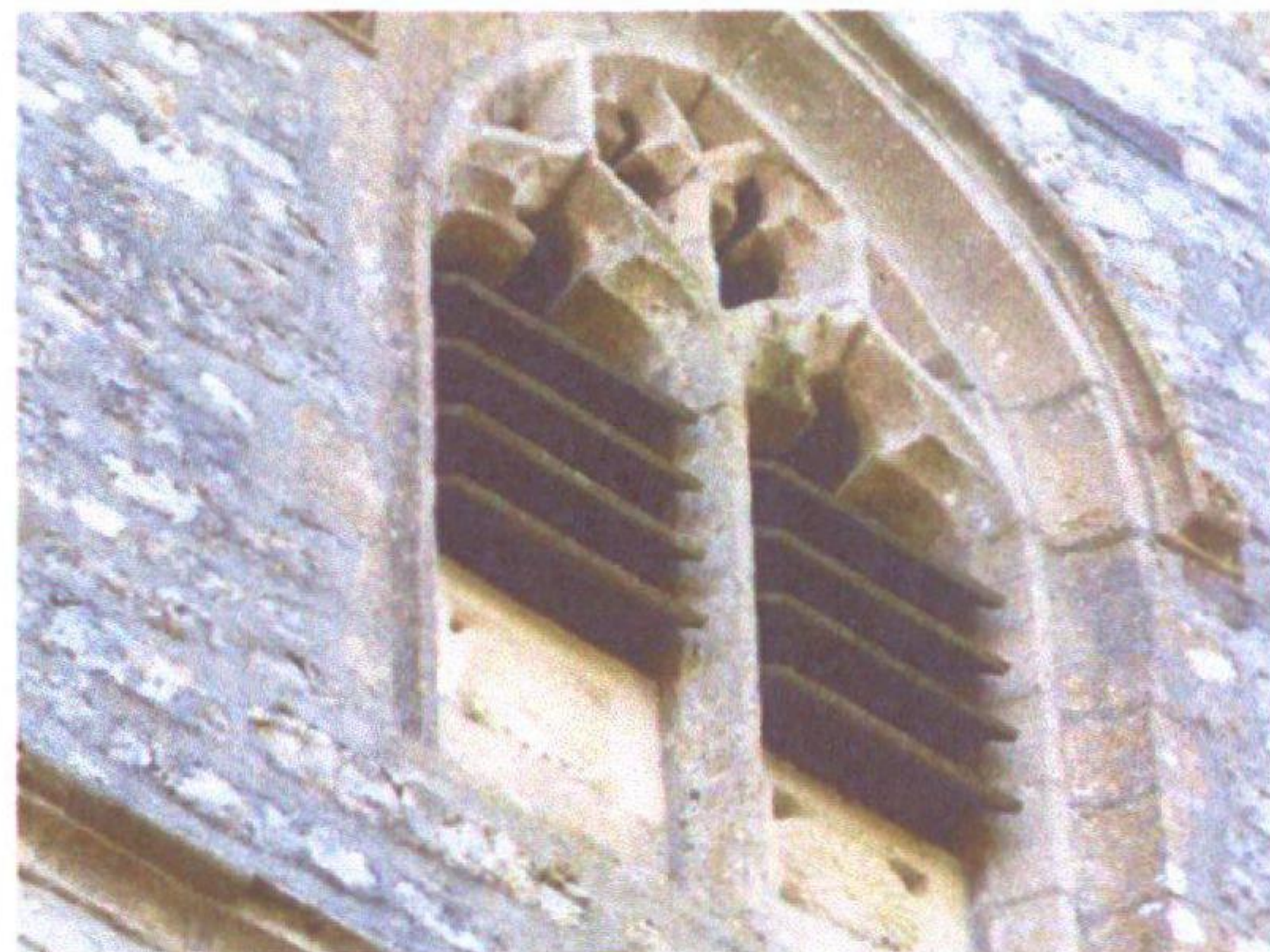
Fig 4 Tower Louvres (Open)
