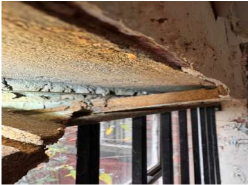
Photograph 5: u1b5-2 Damaged masonry, building interior.
