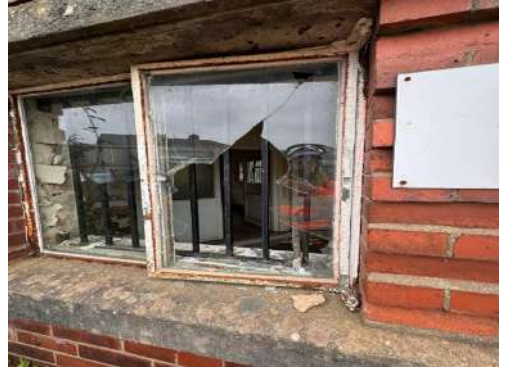
Photograph 4: u1b5-2 Broken window, entry point into the building.
