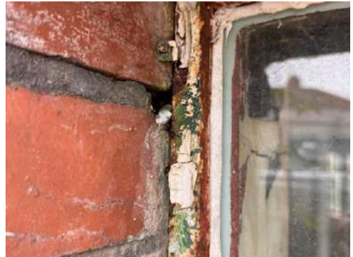
Photograph 6: u1b5-2 Missing mortar, external.
