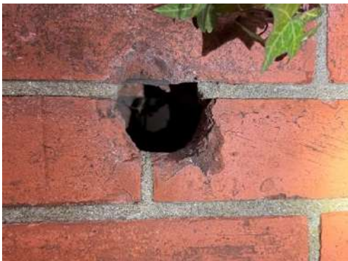
Photograph 7: u1b5-2 Hole within brickwork
