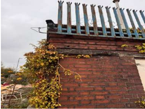
Photograph 3: u1b5-1 Hole within a brick wall.
