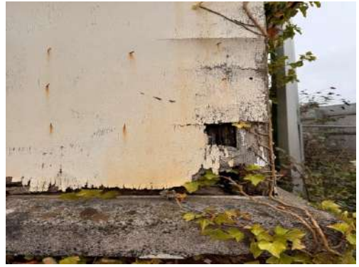
Photograph 2: u1b5-1 Hole within a window board.
