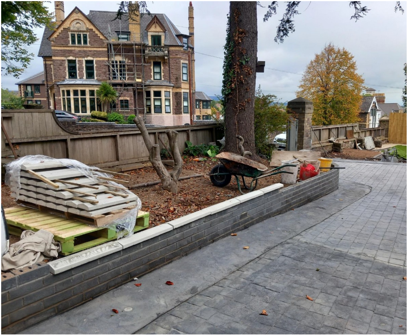
Previously existing arrangement of garden to 46 Caerau Road Road 46 Caerau Road (undertaken without permission)
