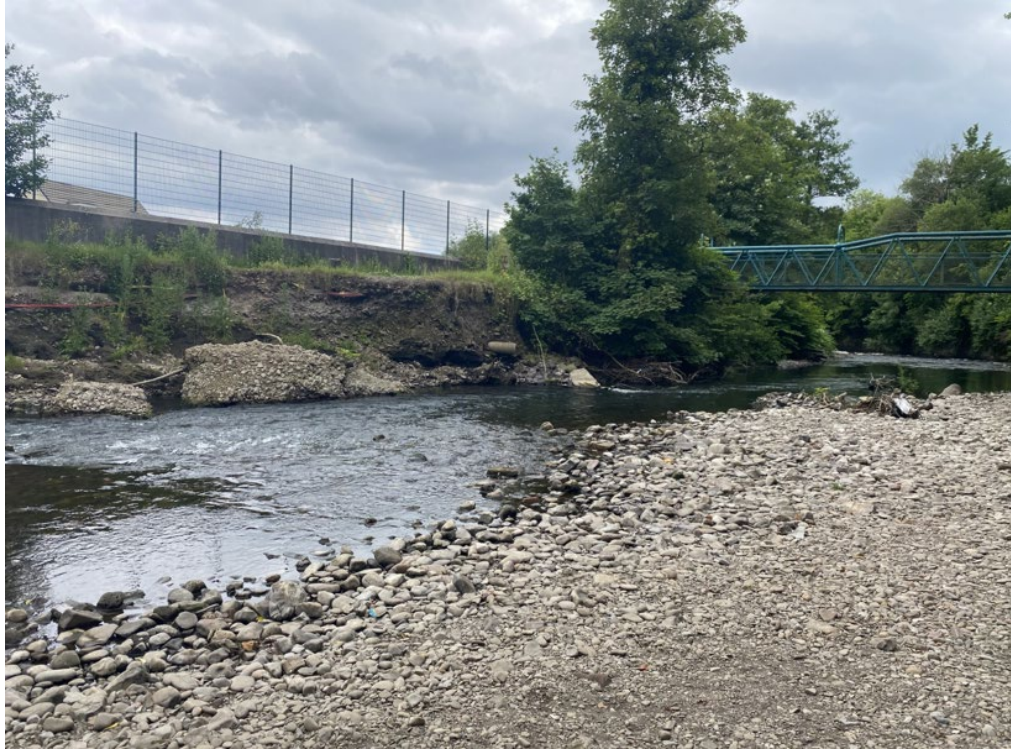
Collapsed bank area on east bank viewed from west
