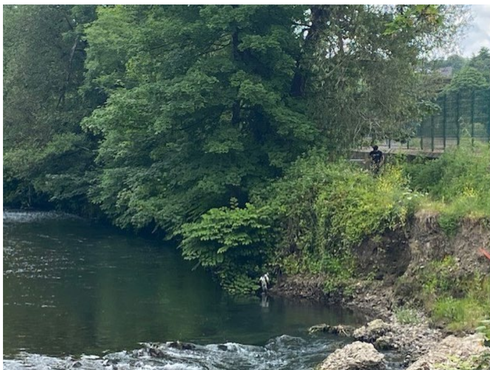
North end of area of collapse illustrating Japanese Knotweed and adjacent bankside trees
