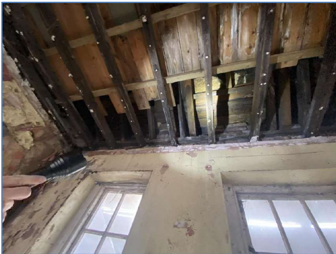
Images 40 and 41 – Second floor, details of damaged ceiling, wall and cornice.
