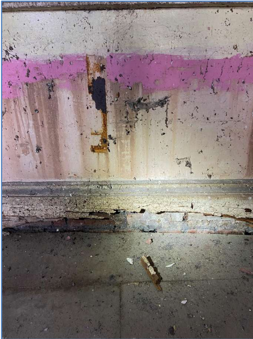
Images 42 and 43 – Second floor, details of damaged wall and cornice.
