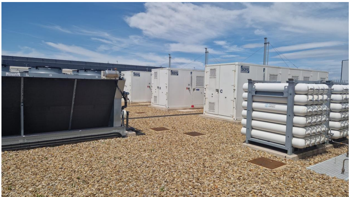
Gas Storage and Compressors
