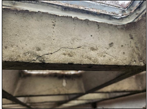
Photograph 8 – Cracking to concrete rooflight frame
