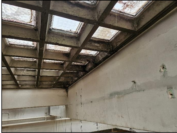
Photograph 7 – Perforations to RC beam
