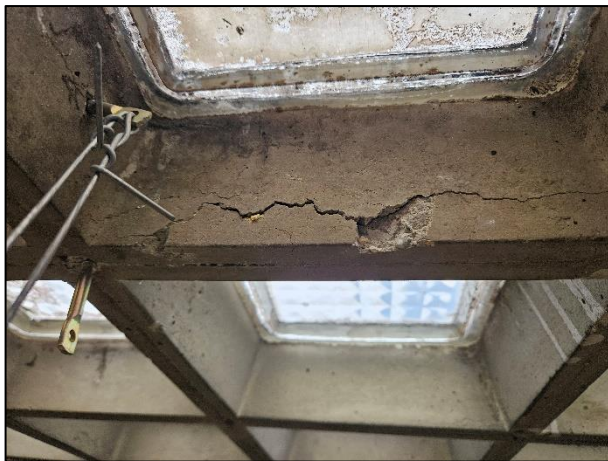
Photograph 9 – Additional cracking to the frame
