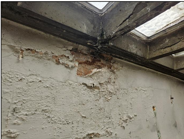
Photograph 3 – Deterioration to main RC beams
