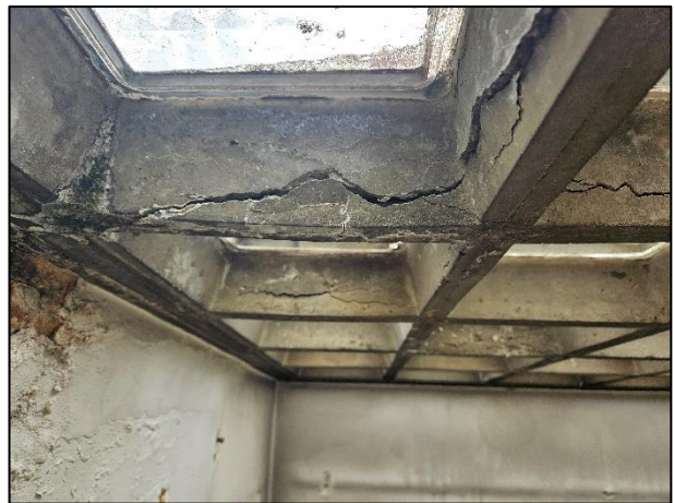
Photograph 10 – Severe cracking to the frame in separate location
