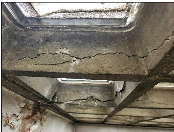
Photograph 11 – Additional noted cracking
