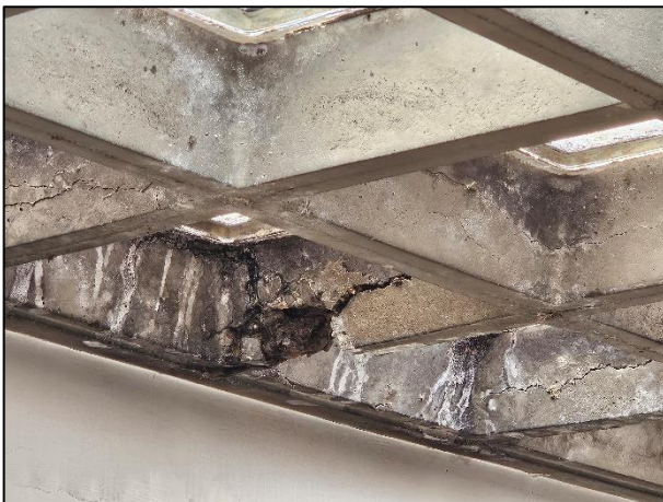
Photograph 5 – Large section of concrete missing from concrete rooflight frame
