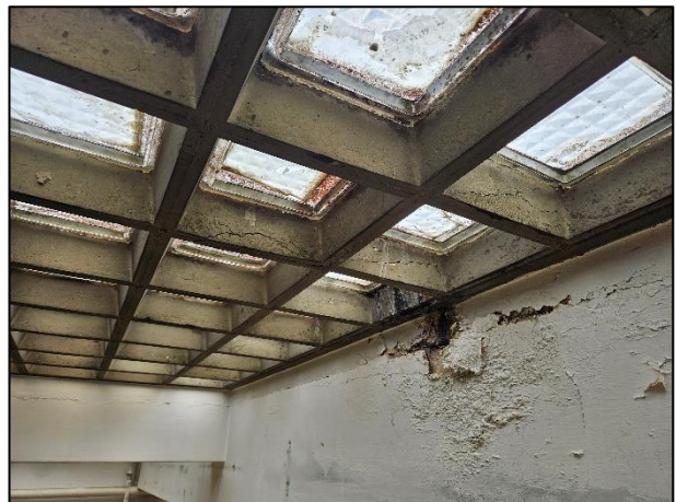
Photograph 6 – Water ingress to main RC beam
