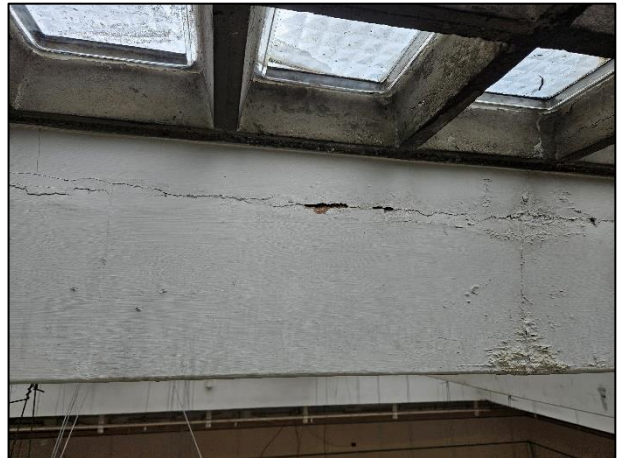
Photograph 16 – Cracking to the RC beam horizontally
