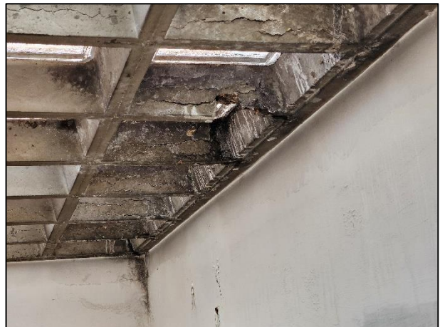
Photograph 18 – Spalling and cracking to Rooflight frame
