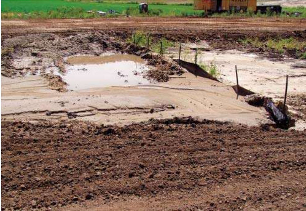
Do not remove sediment. Build a new silt fence for full capacity.
