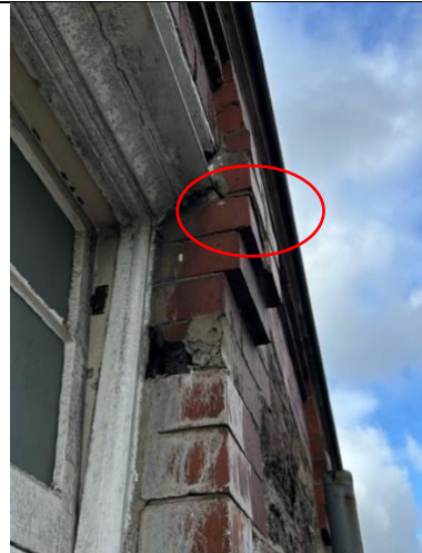
W2 right hand protrusion – slight movement around the beam
