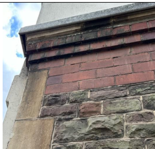
Brick upper courses, rockface stone below with bath stone at the corner junction – discoloured
