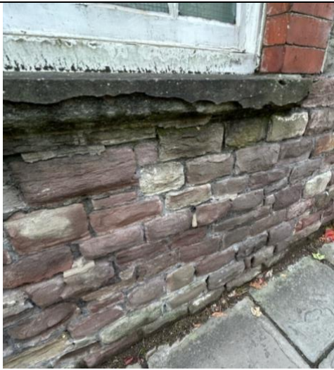
Boys WC (W2) – Delaminating stone cill.
