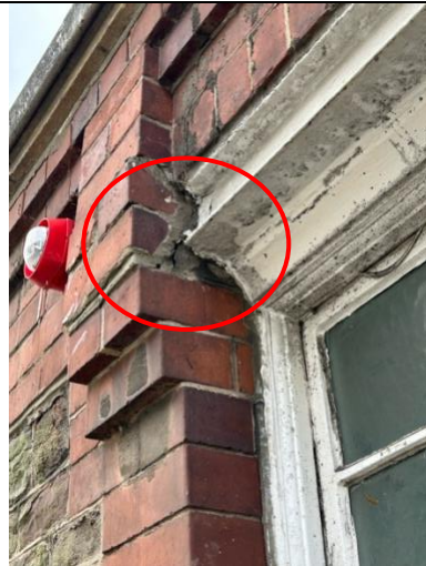
Cracked brickwork and mortar allowing water to track internally
