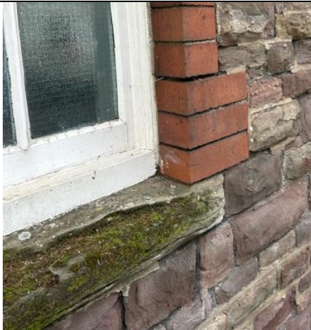
Moss growth to cill – top layers have delaminated
