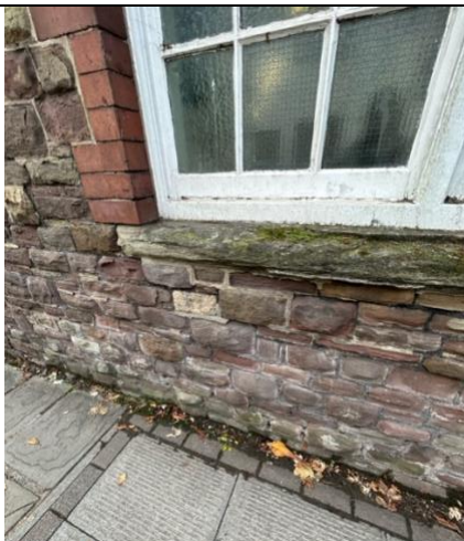
Weathered stonework below cill – colour deterioration from traffic pollution.
