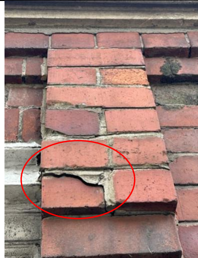
Crack to mortar joint
