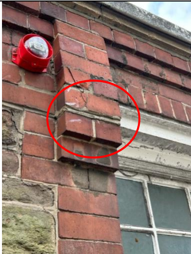
Left stepped protrusion - slight movement of third / forth brick
