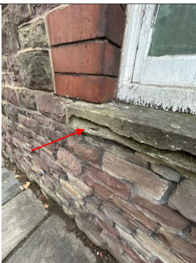
Boys WC (W2) – Delaminating stone cill.
