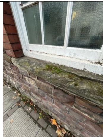
Weathered and deteriorated cill – worse condition out of the three cills. Moss growth to surface, areas becoming porous resulting in further deterioration.
