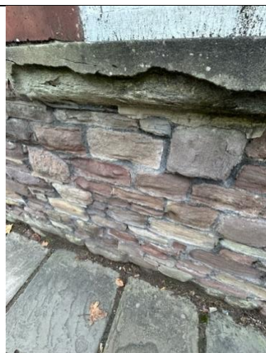
Boys WC (W2) – Delaminating stone cill. Weathered stonework
