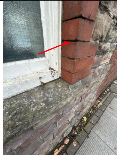
Deterioration of mortar joints – encouraging water ingress internally
