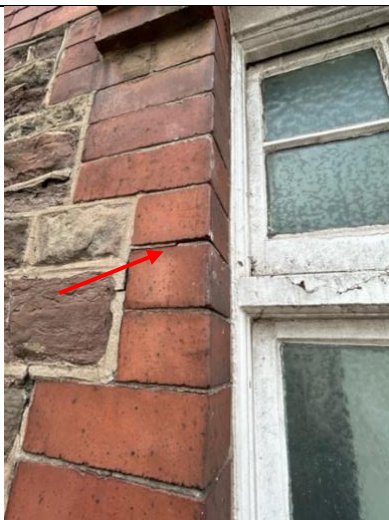
Deterioration of mortar joints in brickwork
