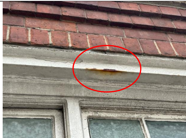
Evidence of spot corrosion to steel beam along edge.
