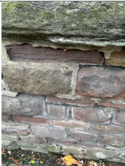
Sand and cement mortar within joints impacting the surrounding stonework.
