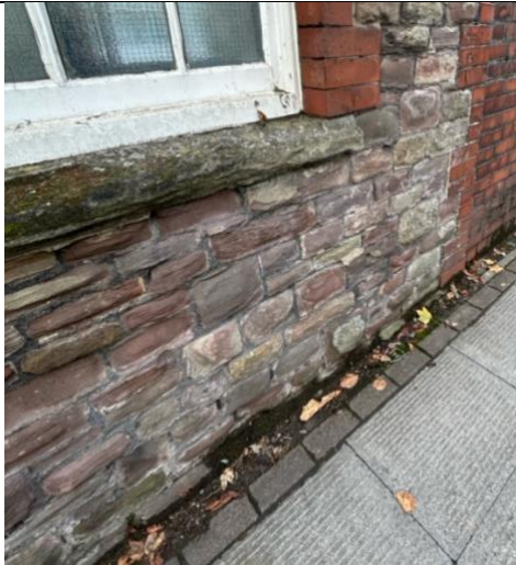
Deteriorated cill – weathered stonework below cill
