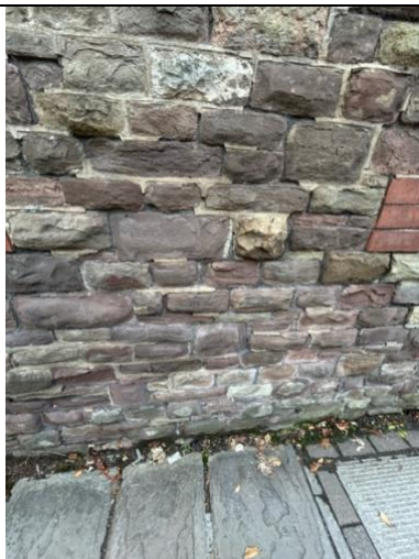
Weathered stonework and mortar joints
