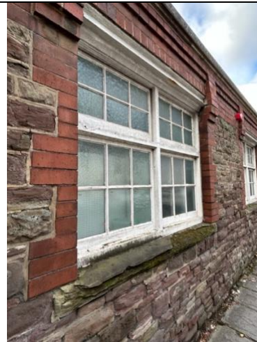
W1 (Girls WC) – Stone cill underside to the left surface crumbling – right side top layer has delaminated
