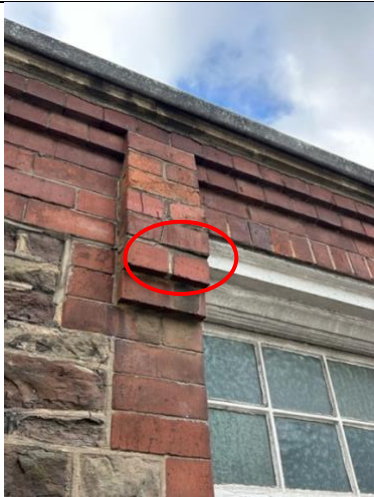
Left stepped protrusion - slight movement of third brick
