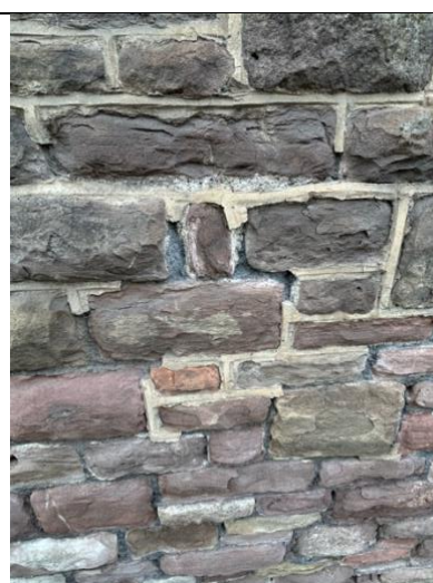
Areas of cement mortar - deteriorated
