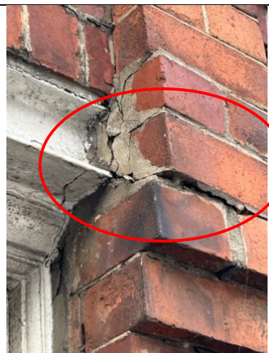
Water sits on the lower lip of the lintel causing water to track between the joints – resulting in further deterioration of lintel and mortar
