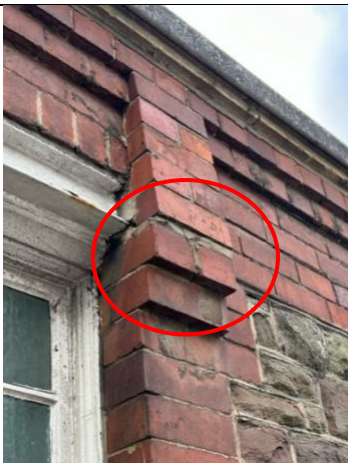
Right stepped protrusion - slight movement of third brick – previous repair to mortar noted. Gaps encouraging ingress at steel lintel junction
