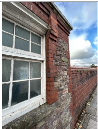
Right stepped protrusion - slight movement of second / third brick
