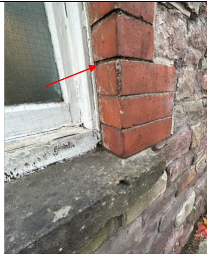
Deterioration of mortar to brick joints.
