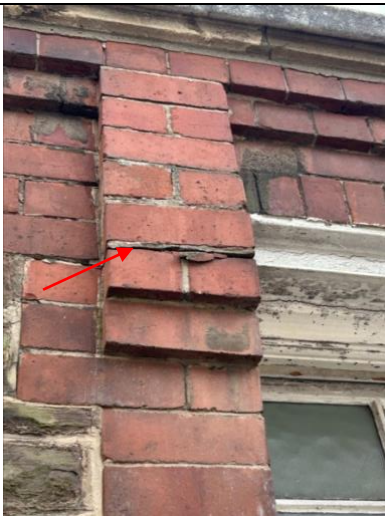
Left window stepped protrusion - brickwork has pushed away from the face of the wall, opening up the joint. Likely due to movement or corrosion of the steel lintel.
