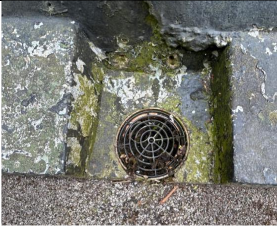
Blocked gully to side / rear elevation to be reviewed further.
