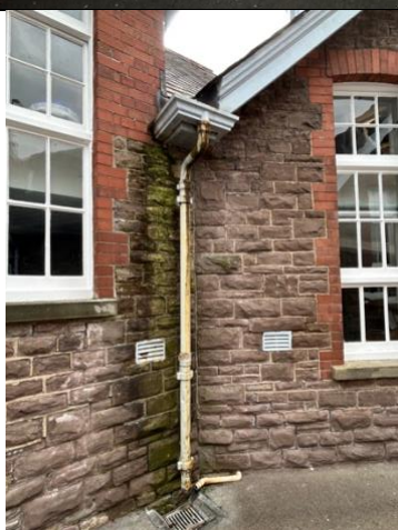
Blocked down pipe causing over spill and damp walls
