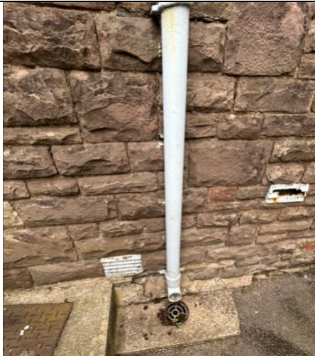
Blocked gully – to be reviewed
