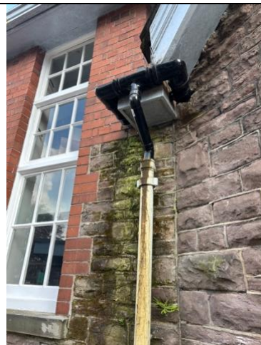
Partial removal – original hopper and bend was completely blocked with debris
