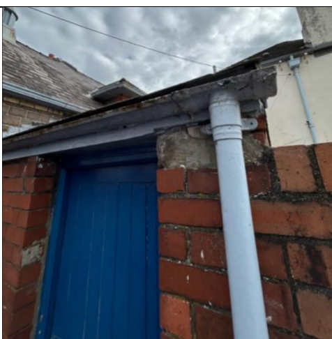
Rain water goods off store room
