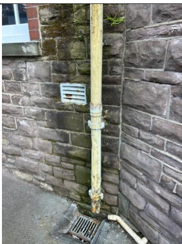
Downpipe remains due to unusual fixings – to be treated on site.
