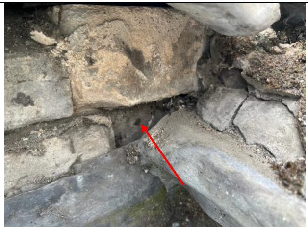
Gaps – potential route for water ingress.
