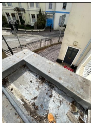
Lead capping – no allowance for expansion
