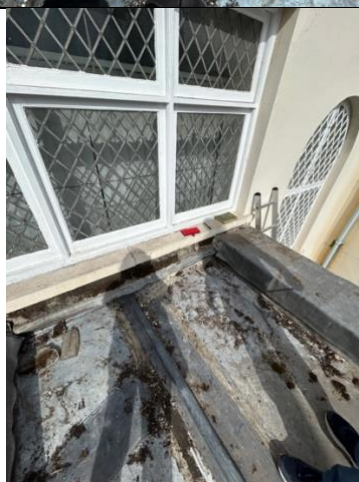
Roof to wall junction – poor detailing
