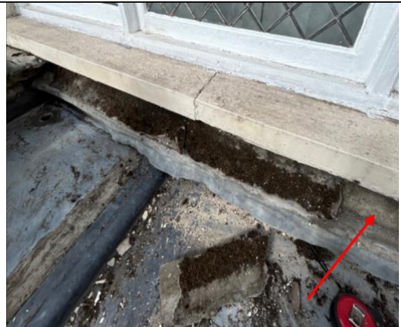
Lead cover flashing not chased into the wall – cement on top has failed
