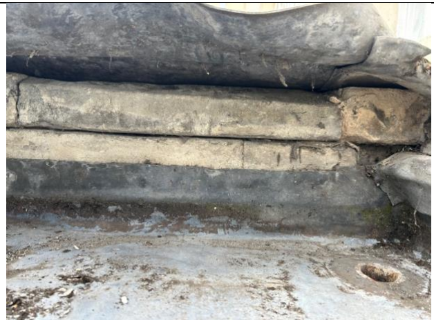
Lead pulled back – capping stones to parapet wall
