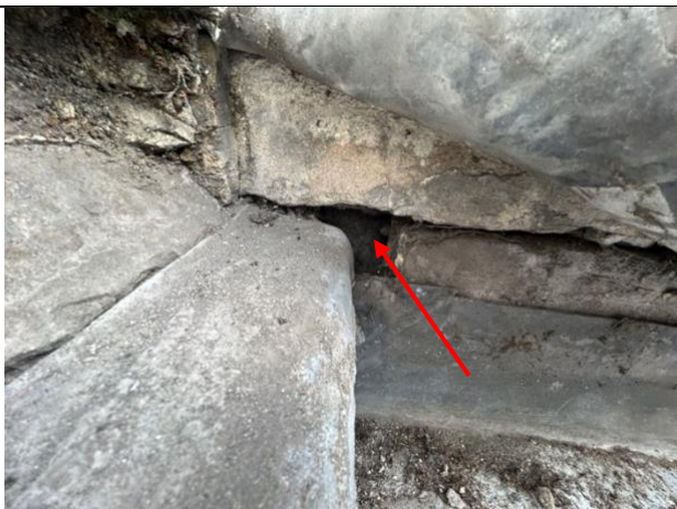
Gaps where lead meets the wall – potential route for water ingress
