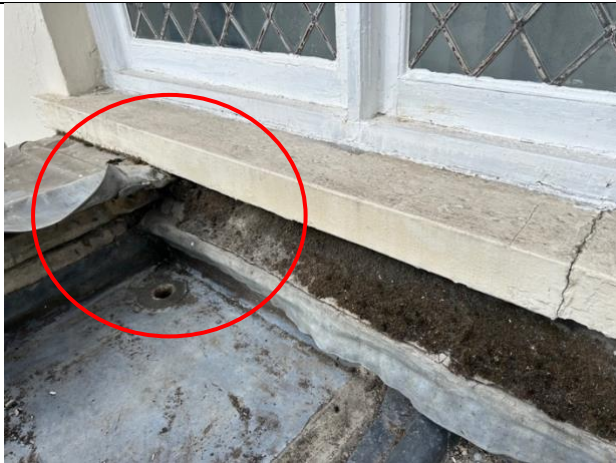
Poor detailing at the corner
