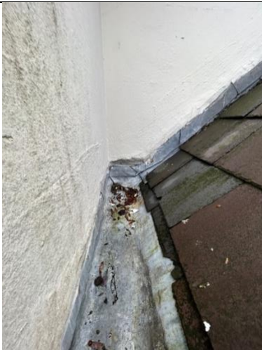
Back gutter to be reviewed and replaced as necessary over the summer.
