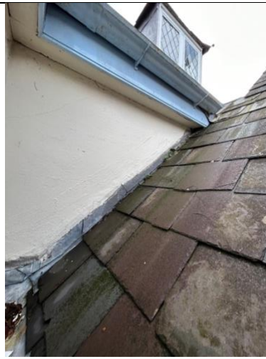
Lead flashing to be reviewed and replaced as necessary
