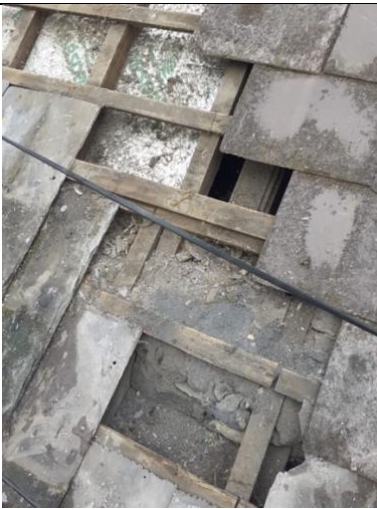
Emergency repairs undertaken over Easter – Deteriorated timber battens and nail fixings.
