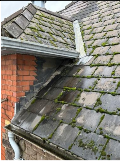
Valley front dormer – potential asbestos slates
