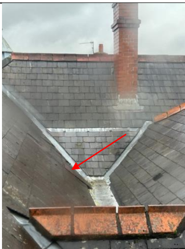
Rear slope to be replaced with New Glendine slate (TBC) – Slates slipped / damaged
