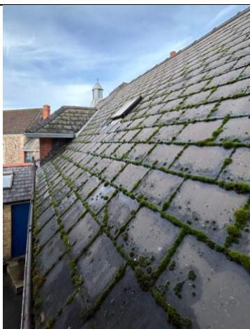
Possibly asbestos slates to part of the roof
