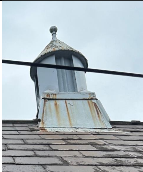
Right slope - currently allowing water ingress to occur into the classroom below.
