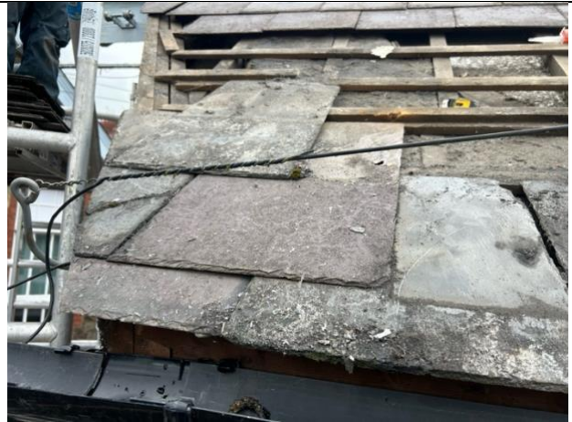
Emergency repairs undertaken over Easter – Deteriorated timber battens and nail fixings.
