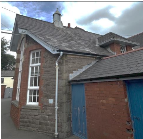
Slope over courtyard – slates have previously slipped – Partial slate roof and slates beyond and including dormer potentially asbestos TBC
