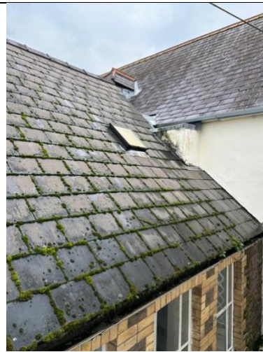
Some areas potentially asbestos slates
