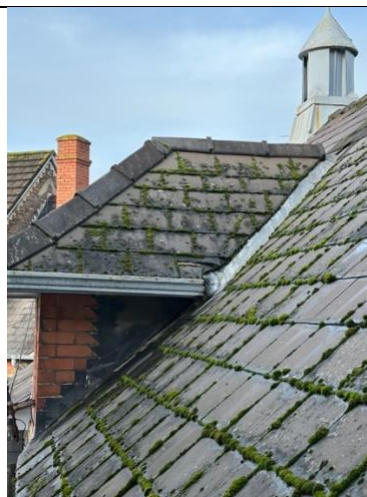
Staffordshire blue ridge or similar to be replaced to match remaining ridge detailing
