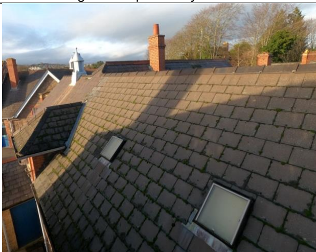
Staffordshire blue ridge or similar to be replaced to match remaining ridge detailing
