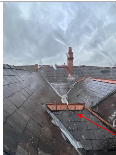
Rear dormer – Slates to be replaced with new – reuse existing ridge / hip tiles – assess lead
