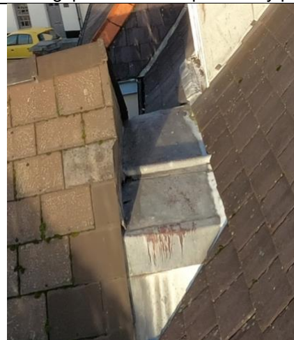
Small lead roof between roof areas – to be reviewed
