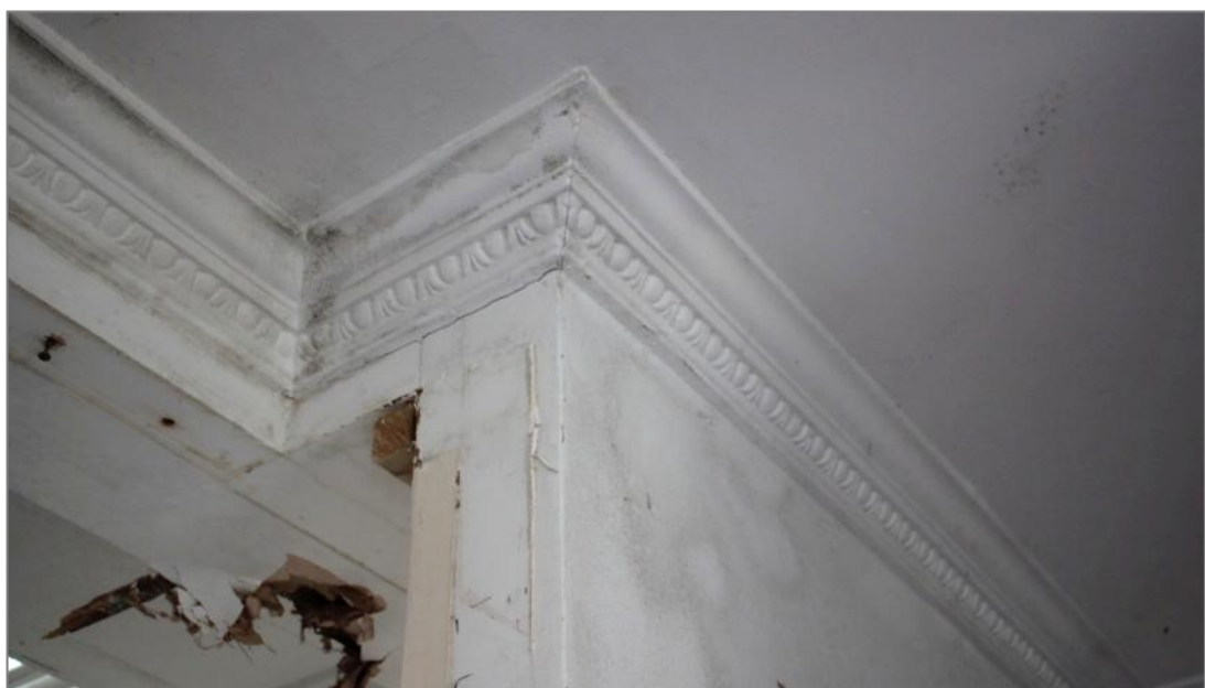
Photo 21: Detail of coving.
