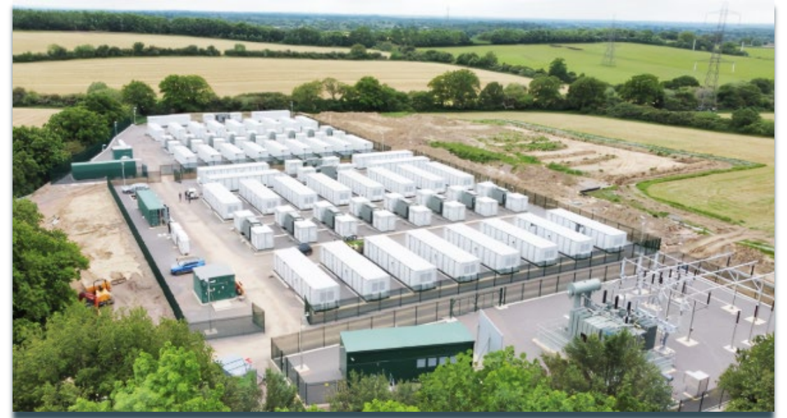
Image of a BESS Facility
