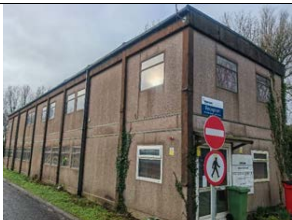
Photo 25: Northern elevation of B4 with dense ivy coverage and vegetation providing sheltered access to roofline and wall junctions
