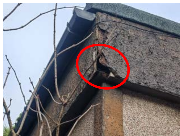
Photo 23: Northern and eastern elevations of B4 with potential gaps along panel joints and roof interface providing possible bat access points
