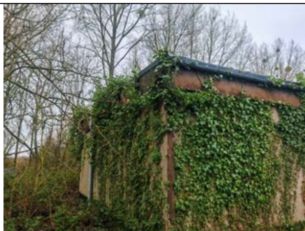
Photo 32: Interface between brick substructure and metal cladding of B6 with ivy growth and roof junctions
