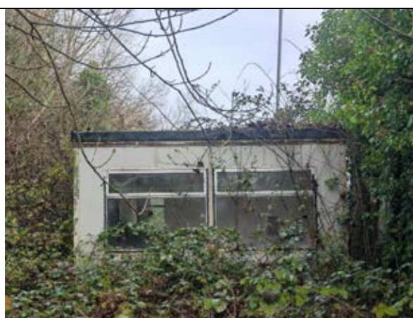
Photo 30: Southern elevation of B5 heavily covered in ivy providing dense vegetative cover and potential access points at roofline and wall junctions
