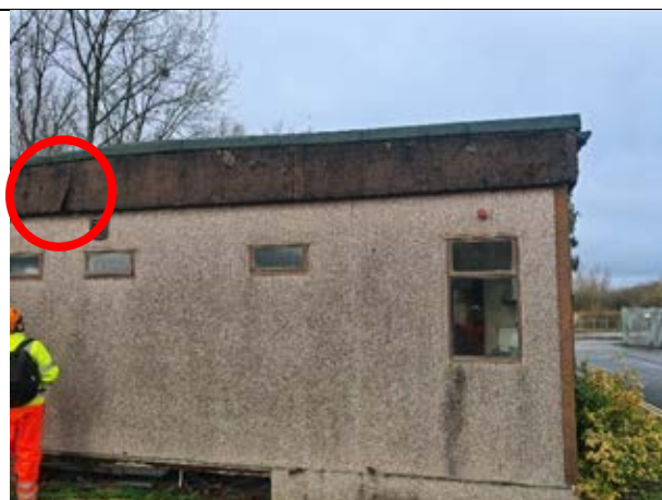
Photo 21: Close-up of roof corner of B3 showing lifted fascia and exposed crevice providing potential bat access
