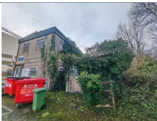
Photo 27: Northern and eastern elevations of B5 showing vegetated margins providing potential crevice opportunities at panel joints and roof interface
