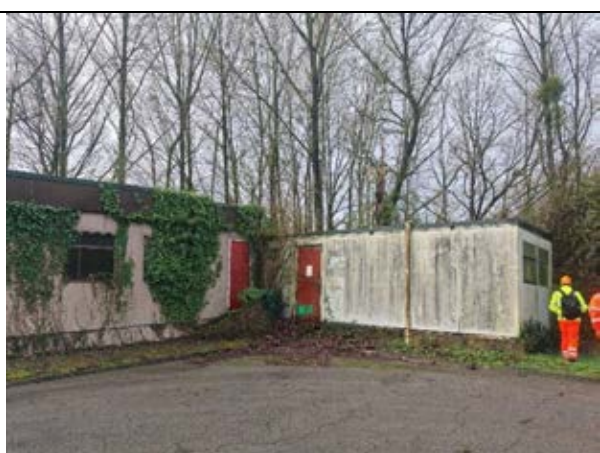
Photo 29: Close-up of damaged soffit and fascia creating lifted boarding and crevice feature beneath roof edge
