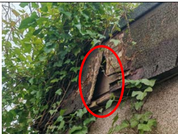
Photo 31: Northern elevation of B6 showing cladding joints and vegetated margins along roofline
