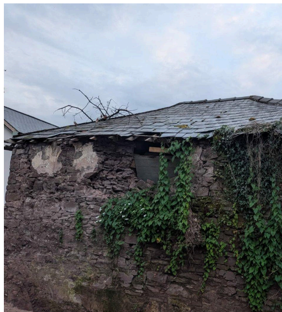
Plate 10 – Rear elevation showing the slate hipped roof with slipped and missing slates, ivy growth and gaps at the eaves/wall junction
