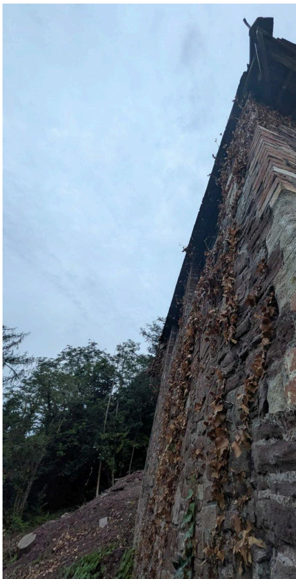
Plate 9 – Rear gable showing exposed stonework, brick quoins, timber rafters at the verge and dead climbing vegetation
