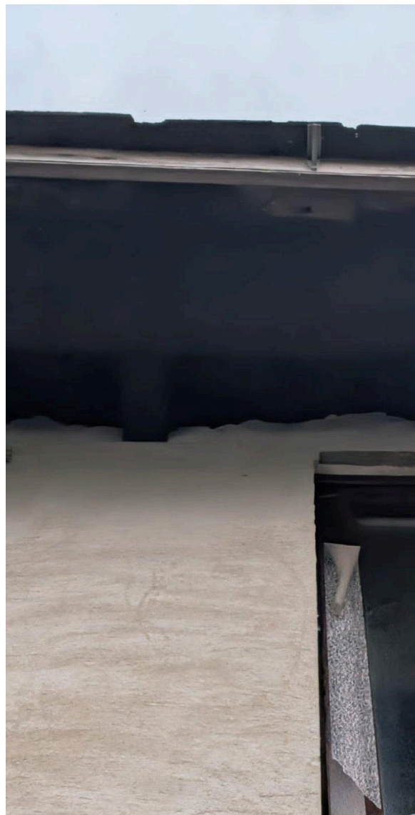
Plate 2 – Eaves and soffit detail showing the painted timber soffit, lead flashing and a gap at the soffit/wall junction
