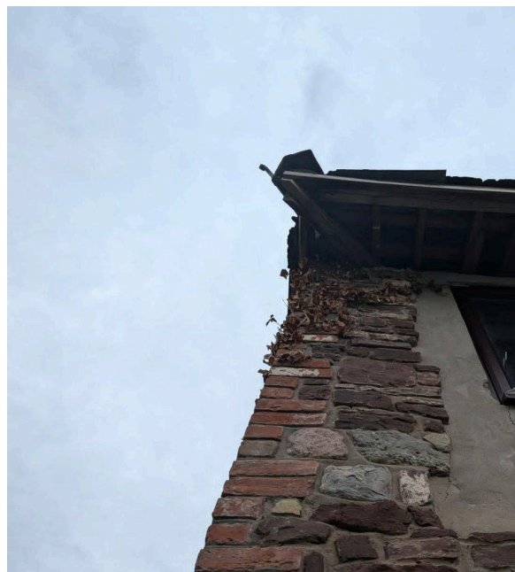
Plate 4 – Gable apex showing exposed random rubble stonework and brick quoins, weathered rafter feet and dead vegetation beneath the eaves
