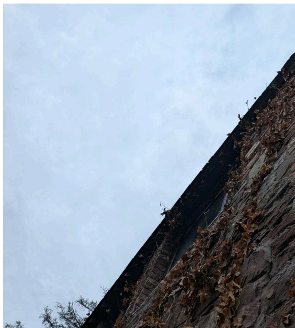
Plate 8 – Gable corner detail showing coursed stone and brick quoins, exposed rafter feet and dead ivy growth beneath the eaves
