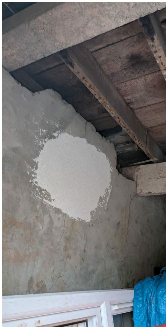
Plate 6 – Ground floor interior showing exposed ceiling joists, cracked render and patched plasterwork to the stone walls
