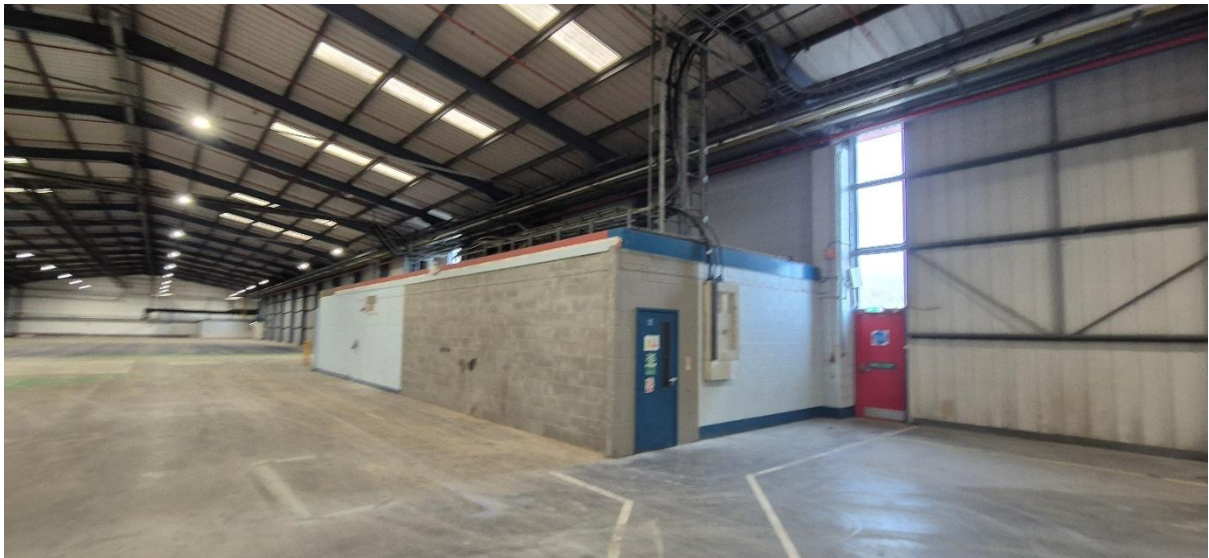
Internal Power Infrastructure
