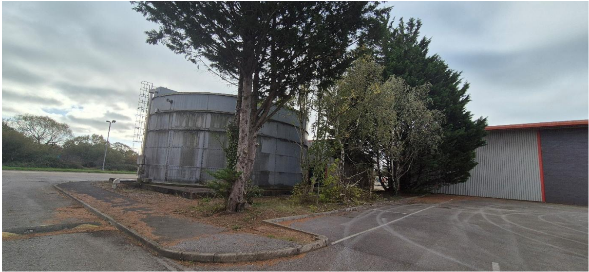
Trees Immediately Adjoining Sprinkler Tank & Warehouse
