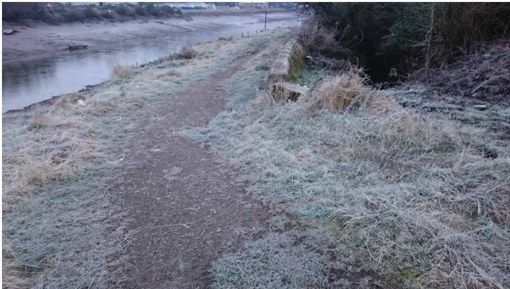
Photo 1-upstream headwall of pipe which passes beneath footpath-outlet situated to the left of photograph
