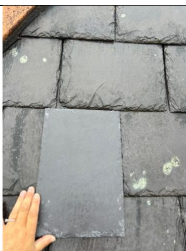
Schoolhouse roof –07.08.25 Wet conditions – NEW penrhyn
