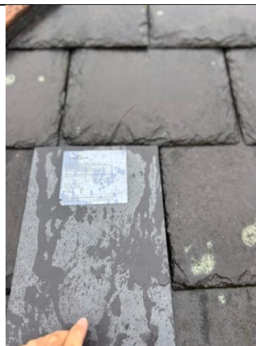
Schoolhouse roof –07.08.25 Wet conditions – NEW penrhyn
