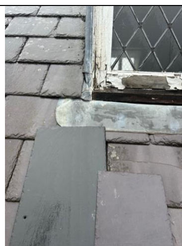
Main schoolhouse – rear slope 07.08.25 Wet conditions – NEW Glendyne and NEW penrhyn
