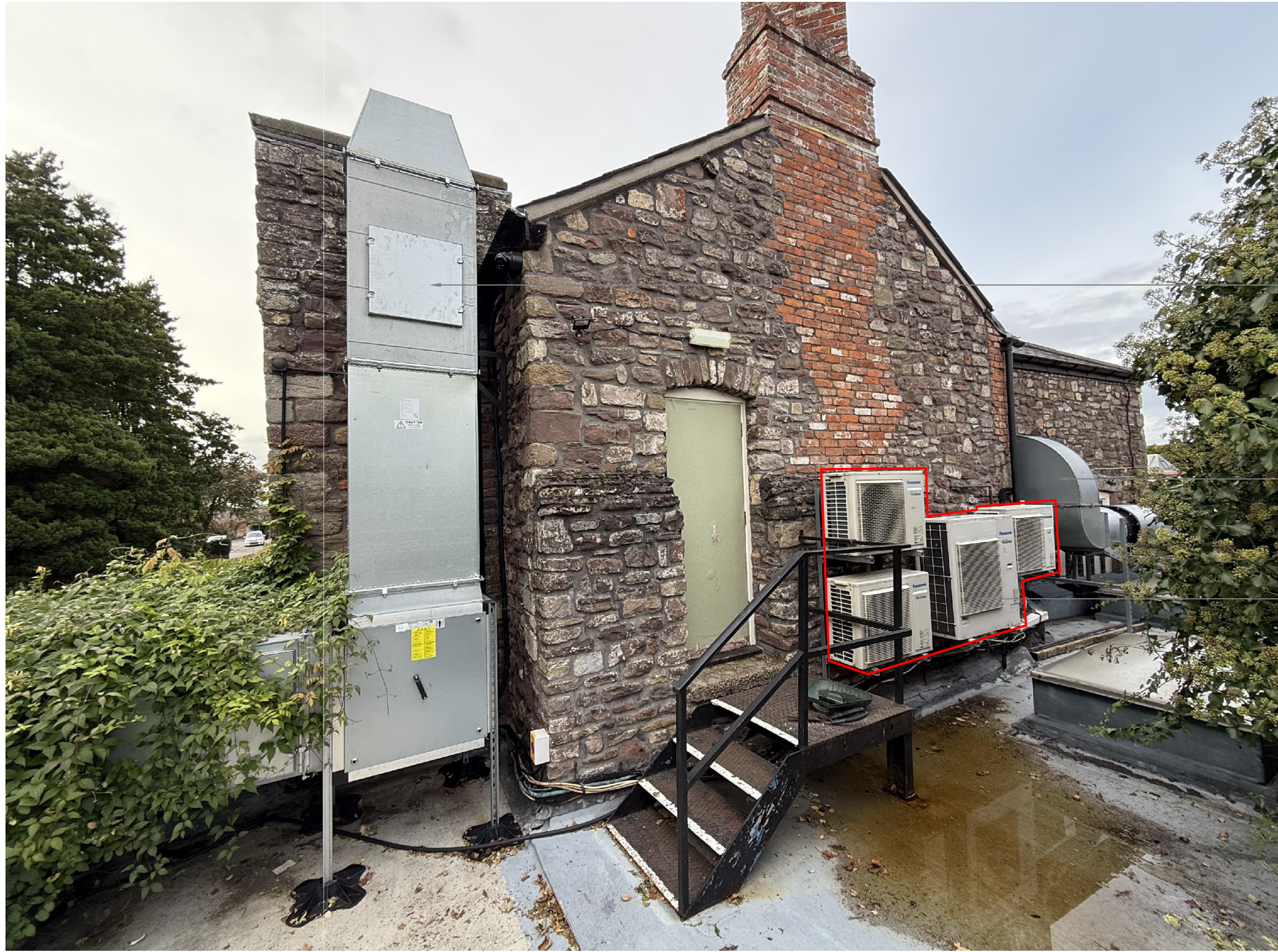
EXISTING LOCATION REFERENCE IMAGE 01 - SHOWING 'PART A' AND 'PART B' EQUIPMENT LOCATIONS VIEW FROM FLAT ROOF (FIRST FLOOR LEVEL)
