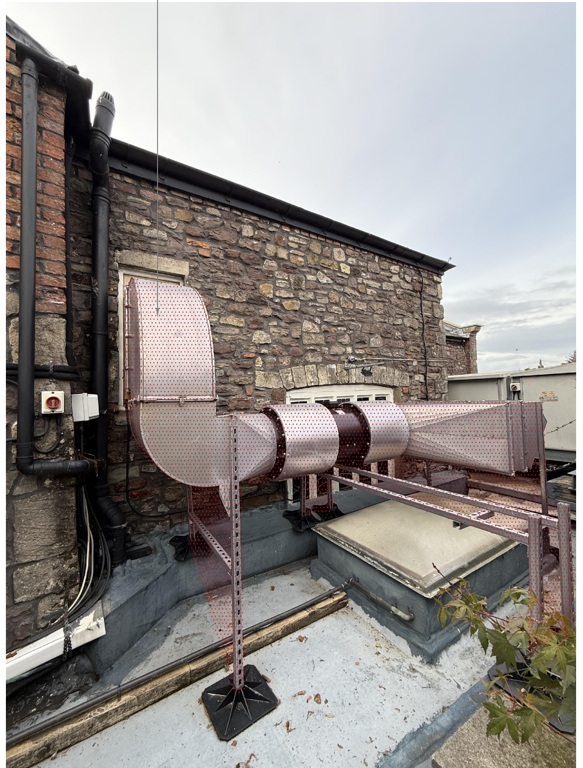
EXISTING LOCATION REFERENCE IMAGE 04 - SHOWING 'PART B' EQUIPMENT VIEW FROM FLAT ROOF (FIRST FLOOR LEVEL)
