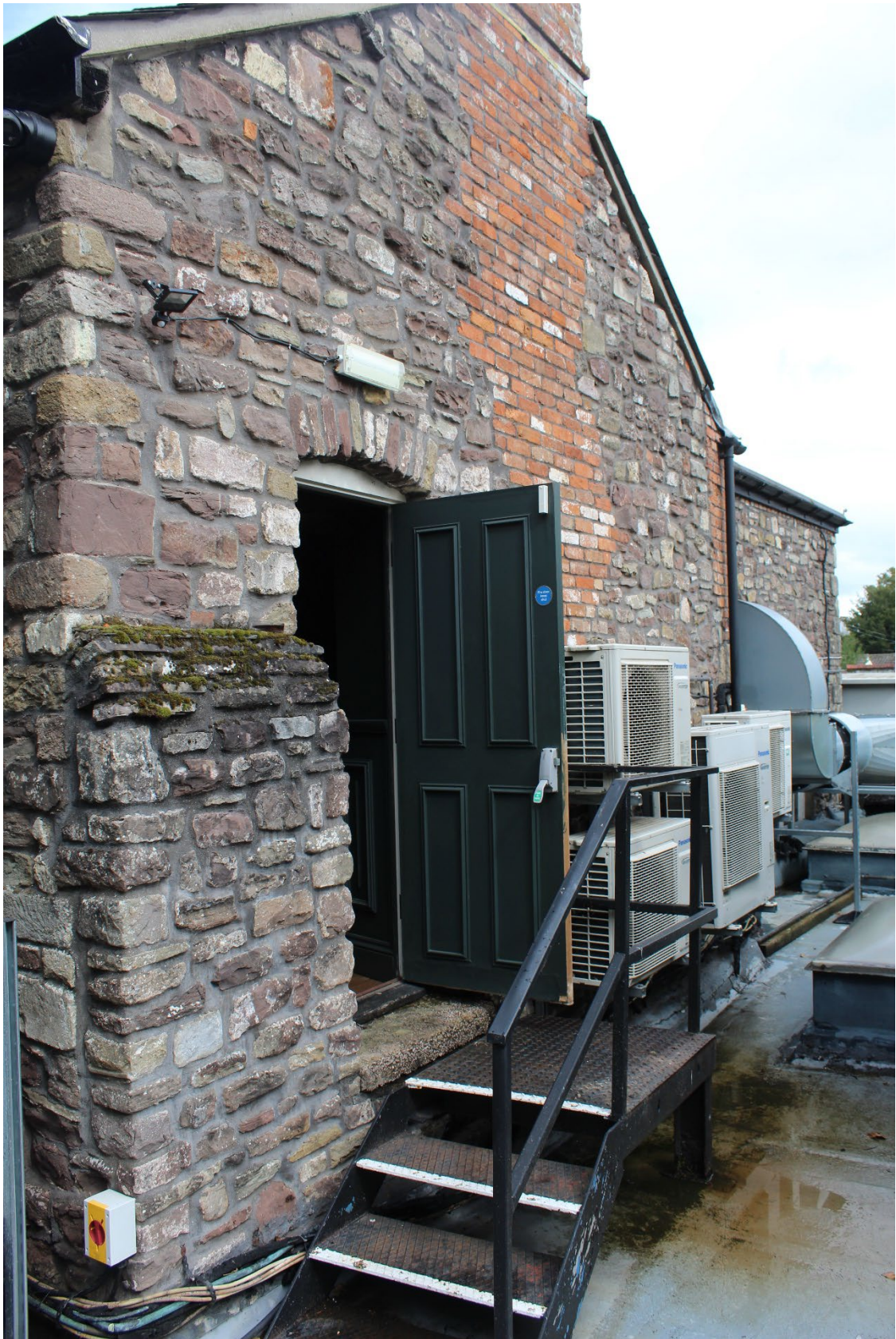
Image EDP A1.18: View of the east end of The Priory and illustrating the locations of the ducts associated with the unauthorised extraction.
