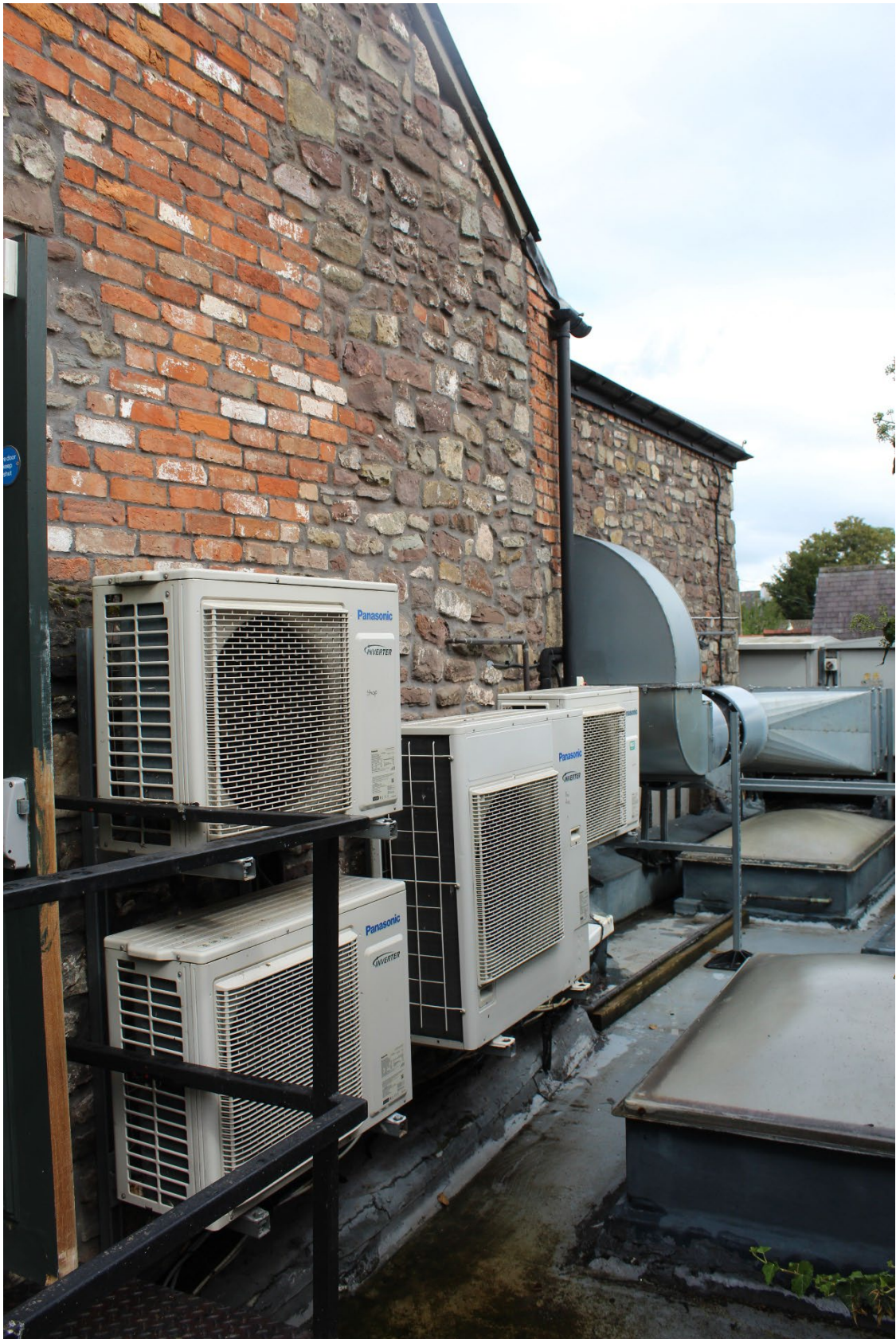
Image EDP A1.9: Close-up of the eastern gable end of The Priory and showing the project site and the unauthorised extraction duct on the eastern elevation of the staircase range.
