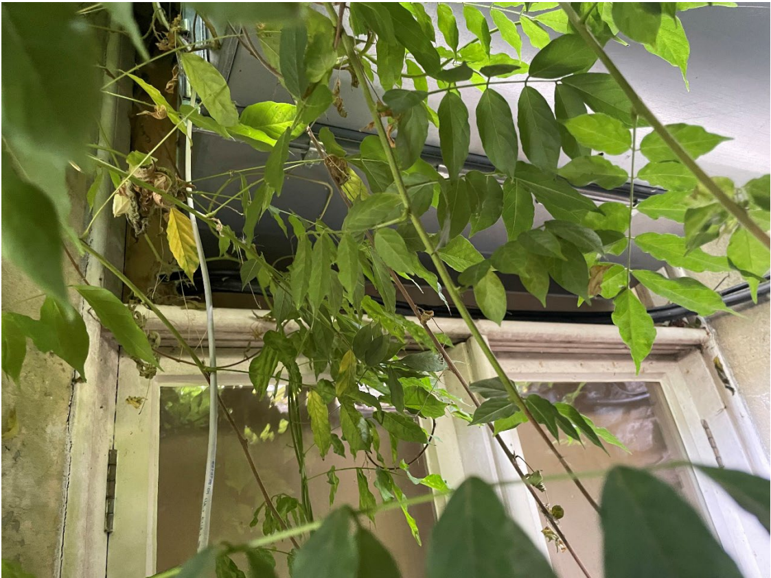
Image EDP A1.15: Close-up of the outside of the window at the south end of the project site and showing the impact of the unauthorised ducting.
