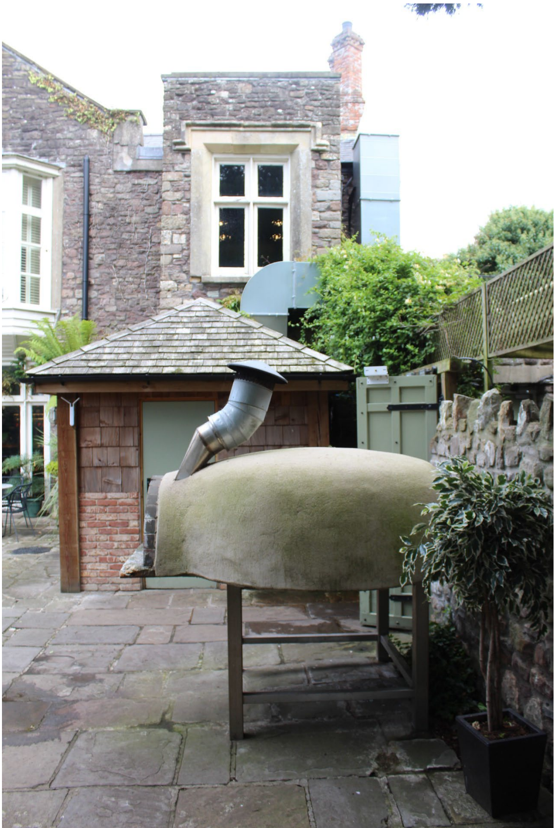
Image EDP A1.8: Close-up of the east end of The Priory from the gardens and showing the project site and the unauthorised extraction duct on the southern elevation.
