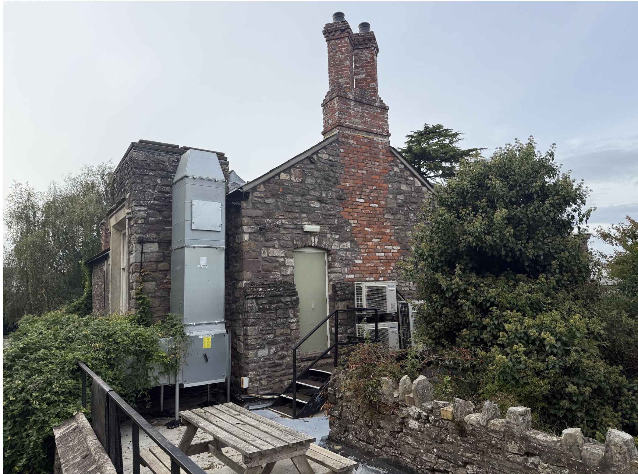
EXISTING LOCATION REFERENCE IMAGE 02 - SHOWING 'PART A' EQUIPMENT VIEW FROM FLAT ROOF (FIRST FLOOR LEVEL)
