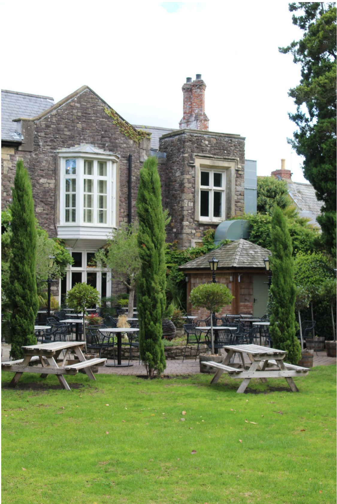
Image EDP A1.7: View of the east end of The Priory from the gardens and showing the project site and the unauthorised extraction duct on the southern elevation.
