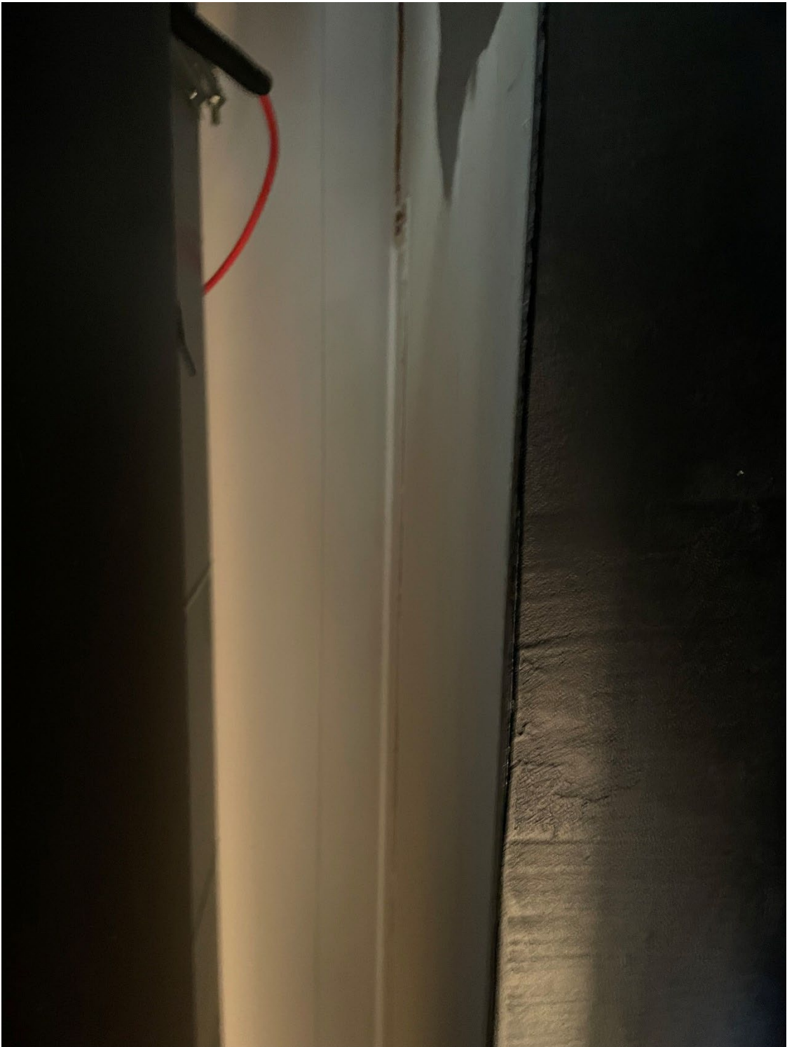
Image EDP A1.13: Close-up of the cornice on the ceiling above the kitchen showing that it is most probably a 20 th century replacement.
