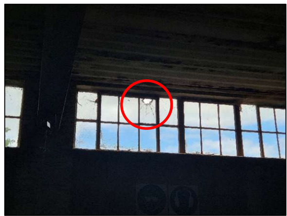
Figure 16 – Damaged Window Pane along (N) Wall of Single-Storey Brick Structure May Permit Access
