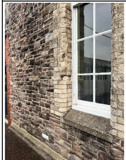
Condition of brick window surrounds SE elevation
