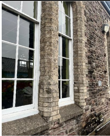
Condition of brick window surrounds SE Elevation
