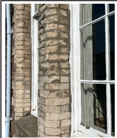
Condition of brick window surrounds SE Elevation
