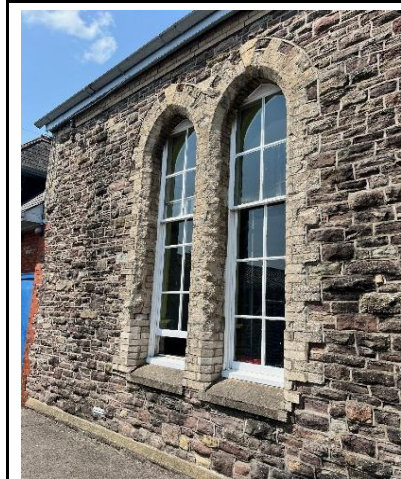
Condition of brick window surrounds SE Elevation
