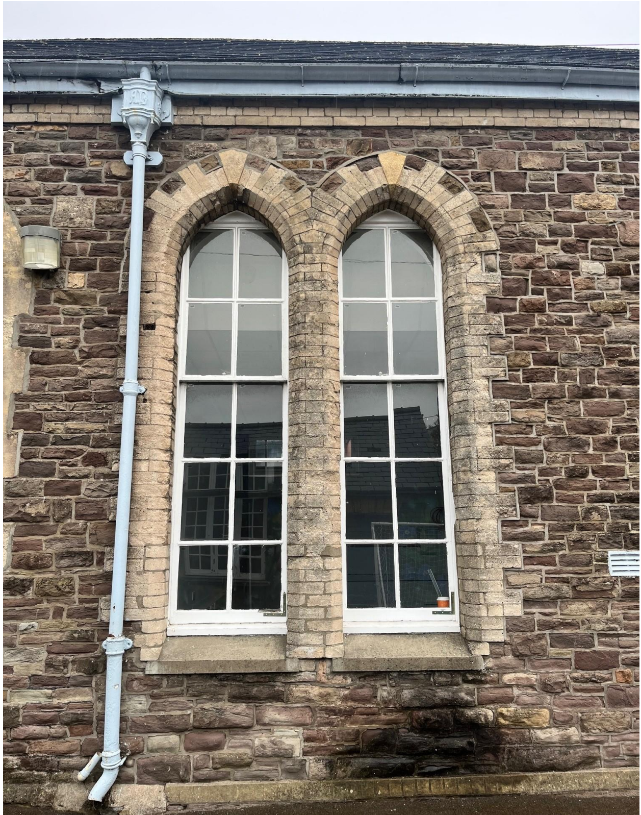
Photo 2: One example of the box sash windows marked for replacement, also condition bargeboards & soffits.
