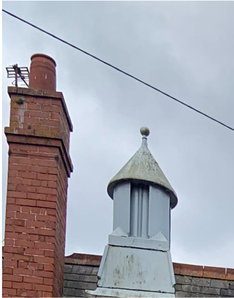
Photo 4: One of two windcatchers marked for maintenance
