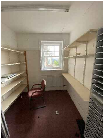
Photo 17: Existing modern type radiator under the window
