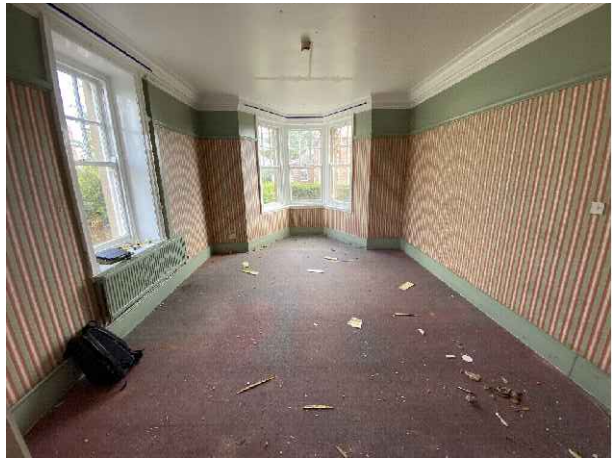
Photo 02: Existing modern type radiator under the window
