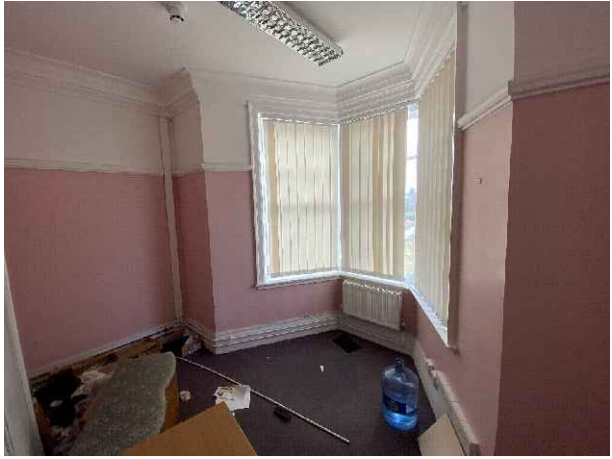
Photo 09: Existing modern type radiator under the window
