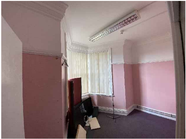
Photo 10: Existing modern type radiator under the window behind the rubbish
