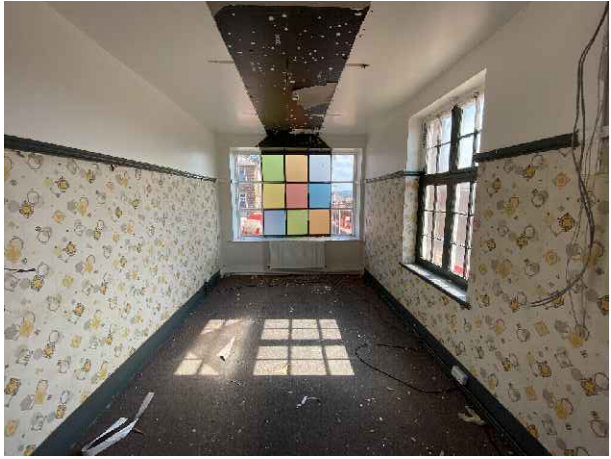
Photo 05: Existing modern type radiator under the window
