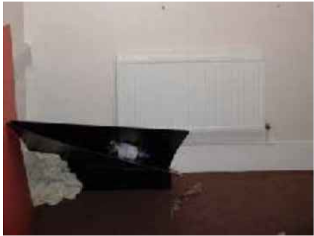
Photo 04: Existing modern type radiator
