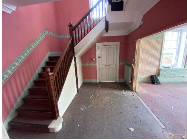
Photo 01: Existing modern type radiator by front entrance door
