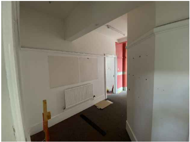
Photo 06: Existing modern type radiator in hallway
