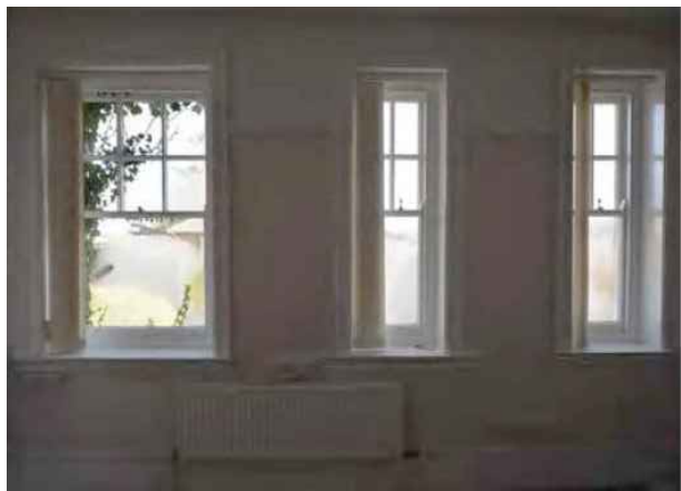
Photo 14: Existing modern type radiator under the window
