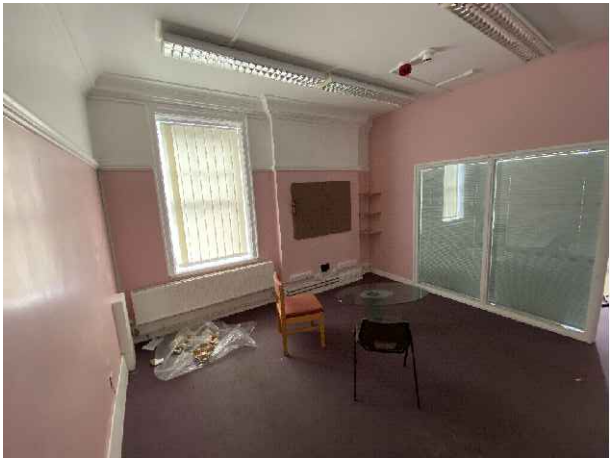
Photo 08: Existing modern type radiator under the window
