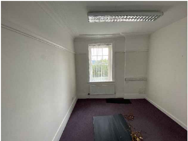
Photo 18: Existing modern type radiator under the window
