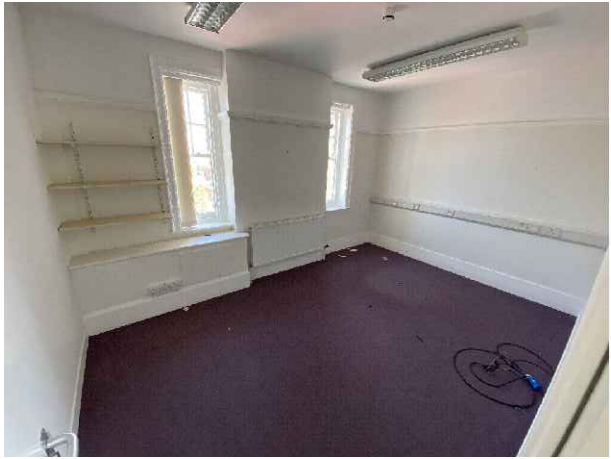
Photo 15: Existing modern type radiator under the window
