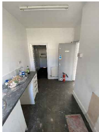
Photo 03: Existing modern type radiator behind the door
