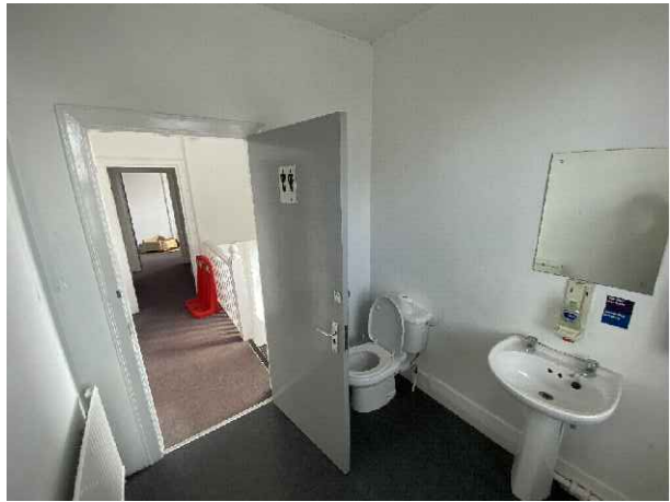
Photo 04: Existing modern type radiator by door way
