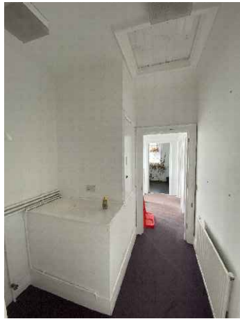
Photo 09: Existing modern type radiator by door way
