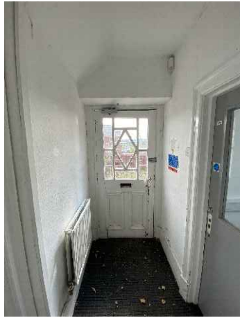
Photo 01: Existing modern type radiator by front entrance door
