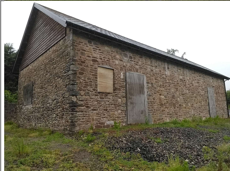
Photo 2. Northwest elevation also with missing glazing in the second floor.
