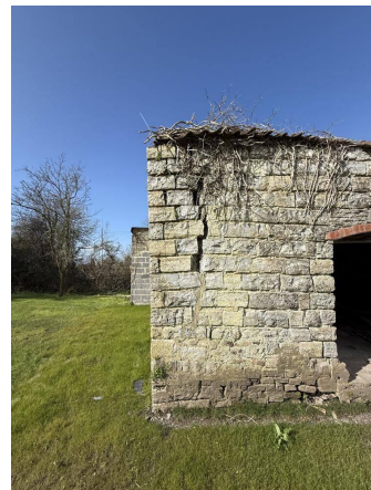
Plate 4. South gable of the stone outbuilding, showing the substantial vertical crack opening to approximately 80 mm at the parapet (see paragraph 5.4.2).
