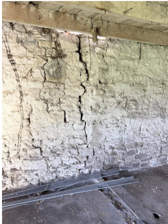
Plate 9. Internal continuation of the south-gable vertical crack, with timber lintel above. To be addressed through stabilisation and partial rebuild (see paragraph 7.3).
