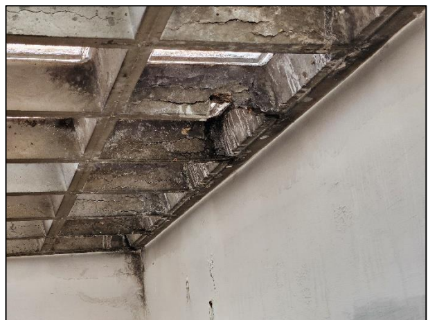
Photograph 18 – Spalling and cracking to Rooflight frame
