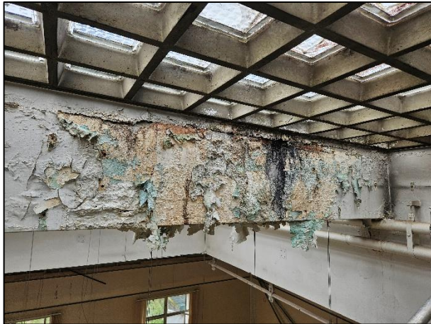
Photograph 13 – Further section on main RC beam damage
