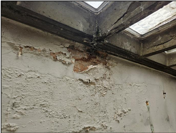
Photograph 3 – Deterioration to main RC beams
