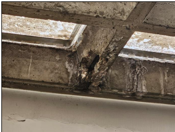
Photograph 15 – Close up of spalled area concrete from rooflight frame
