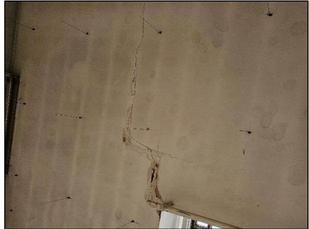
Photograph 14 – Diagonal cracking propagating window to roof
