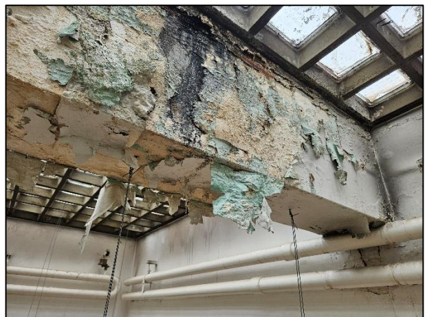
Photograph 12 – Large deterioration to main RC beam exterior
