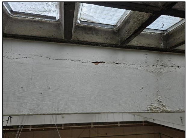
Photograph 16 – Cracking to the RC beam horizontally
