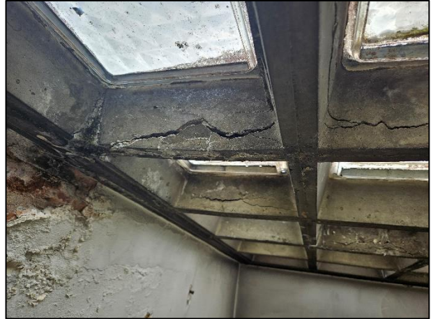
Photograph 2 – Close up of cracking to concrete supporting frame
