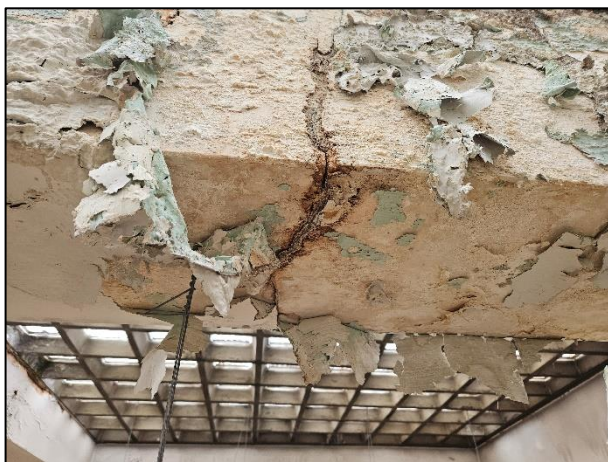
Photograph 17 – Large crack in RC beam up close
