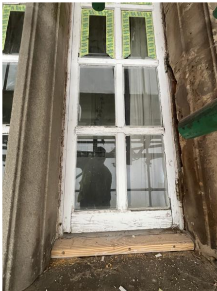
Plate 4: Window W01 Prior to pointings
