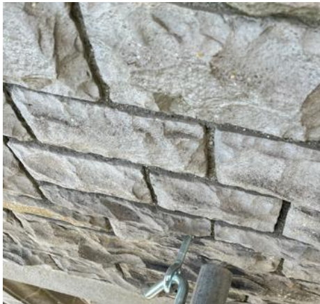
Plate 1: Existing pointings (lias panels)
