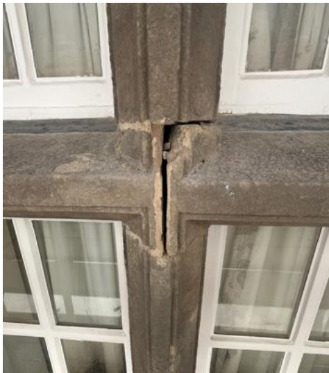
Plate 1: Existing stone cracking / parting
