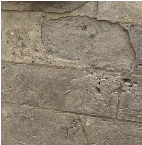
Plate 1: Existing stone face delaminations
